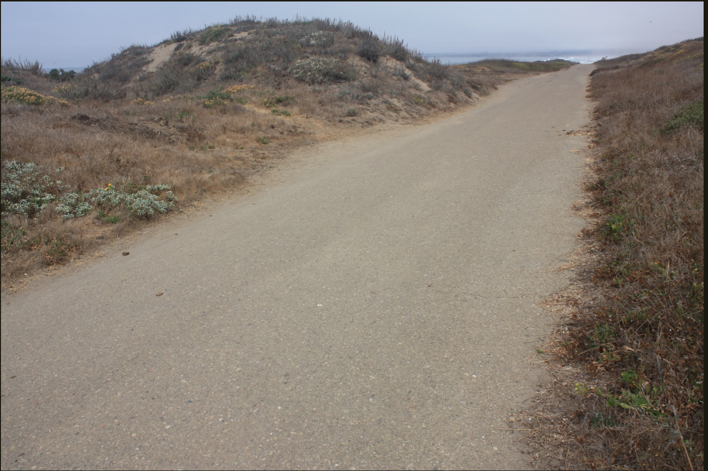
Northwestward view of the TM (1916), 3 miles north of the previous location and 4 miles north of Fort Bragg. The paved surface is the 1954 haul road; Pacific Ocean in the distance. Note the sand dunes on which the grade is built; the northern half of the TM (1916) is built on coastal dunes.
