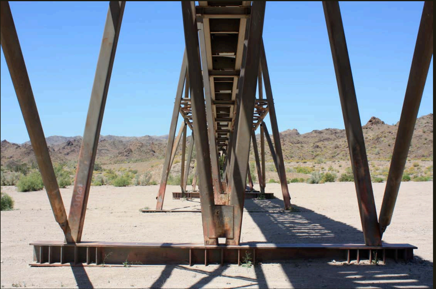
The EMRR Salt Creek Wash Bridge has no pilings or foundation in the riverbed; instead, the bridge “floats” on the sandy the wash.
