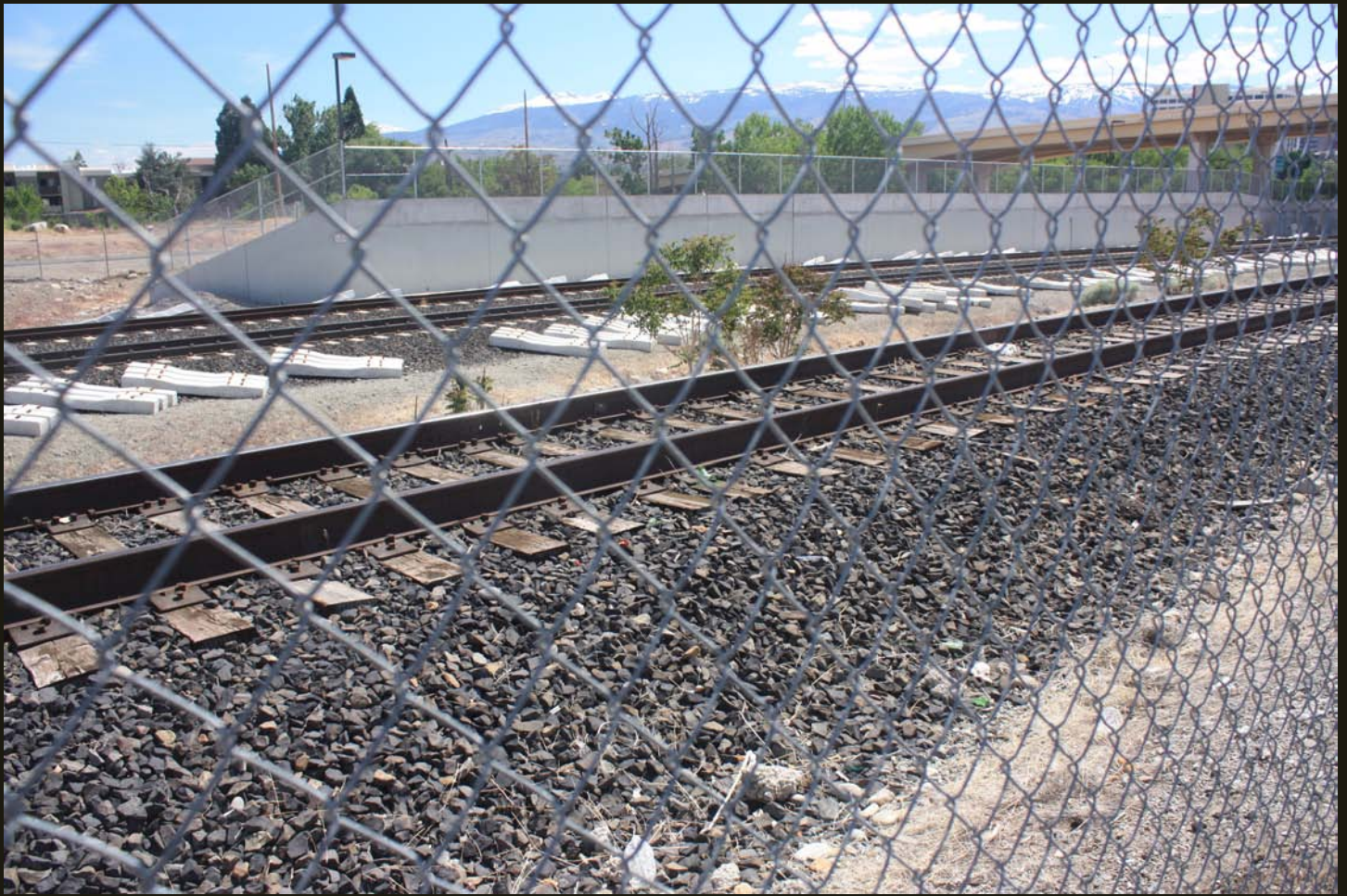
Southwestward view of the CP (1869), represented by the two distant tracks with concrete ties, in the center of the 2,700-foot siding, represented by the track with wooden ties in the foreground. The white retaining wall is the east end of the ReTRAC lowering of the grade through downtown Reno.
