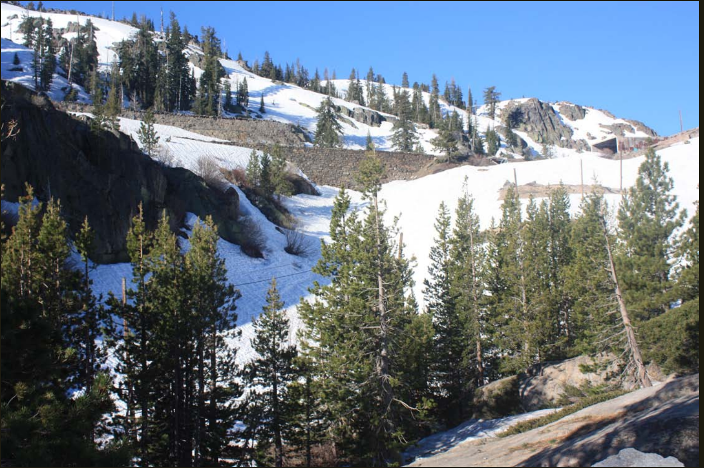
Southward view of the China Wall. Rock excavated from the summit tunnel was used to fill in the ravine and was faced with perfectly fitted quarried granite; there is no mortar in the cracks. The upper wall protects the track from avalanches and slides. The walls are in perfect condition, looking good for 150 years old and more than a century of heavy rail traffic.
