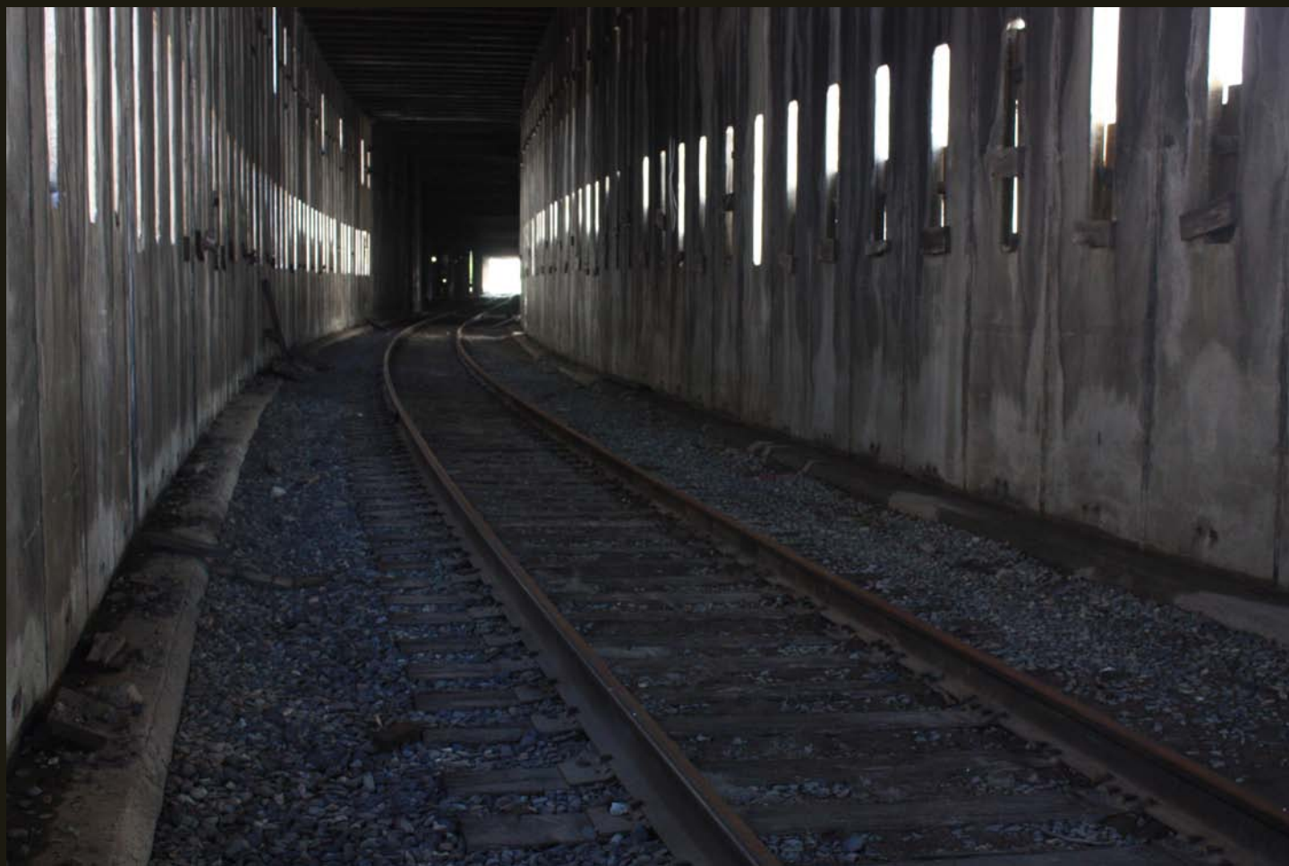
Westward view of the west shed entrance, the light at the end of the tunnel in this view. The original (1867) CP alignment, which is the northernmost of the three eastern entrances, is in the foreground.
