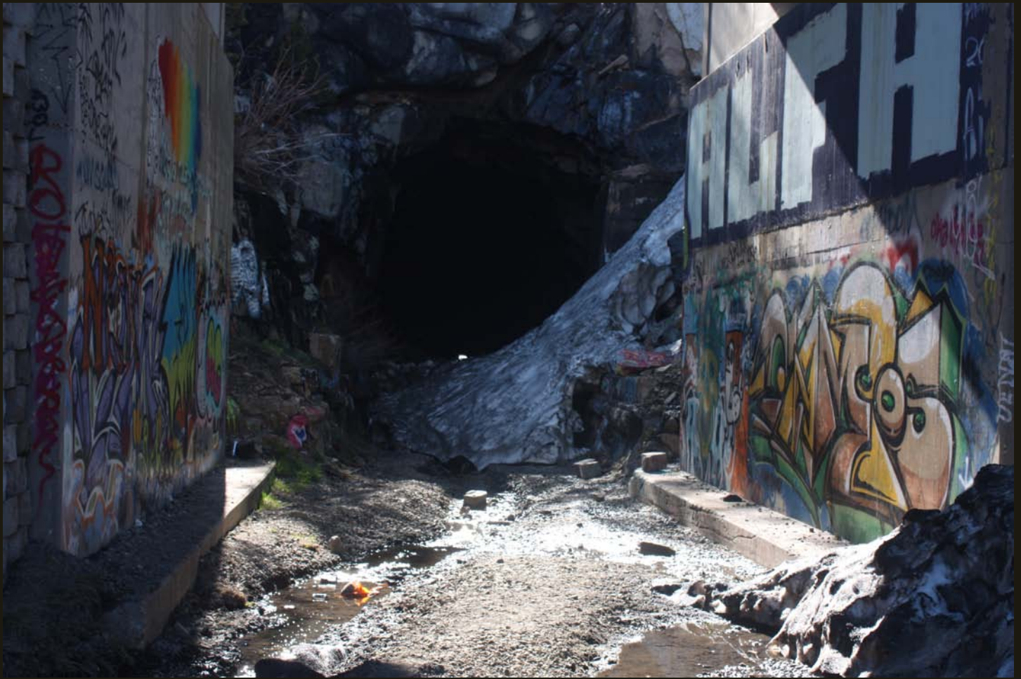
Eastward view of the west entrance of the original CP summit tunnel, built by thousands of Chinese craftsmen and laborers during 1867 and 1868. The graffiti covered retaining walls support Sugar Bowl Road. Note that the 1,659-foot tunnel has no concrete work, which was not needed because the glaciated granite is so hard.
