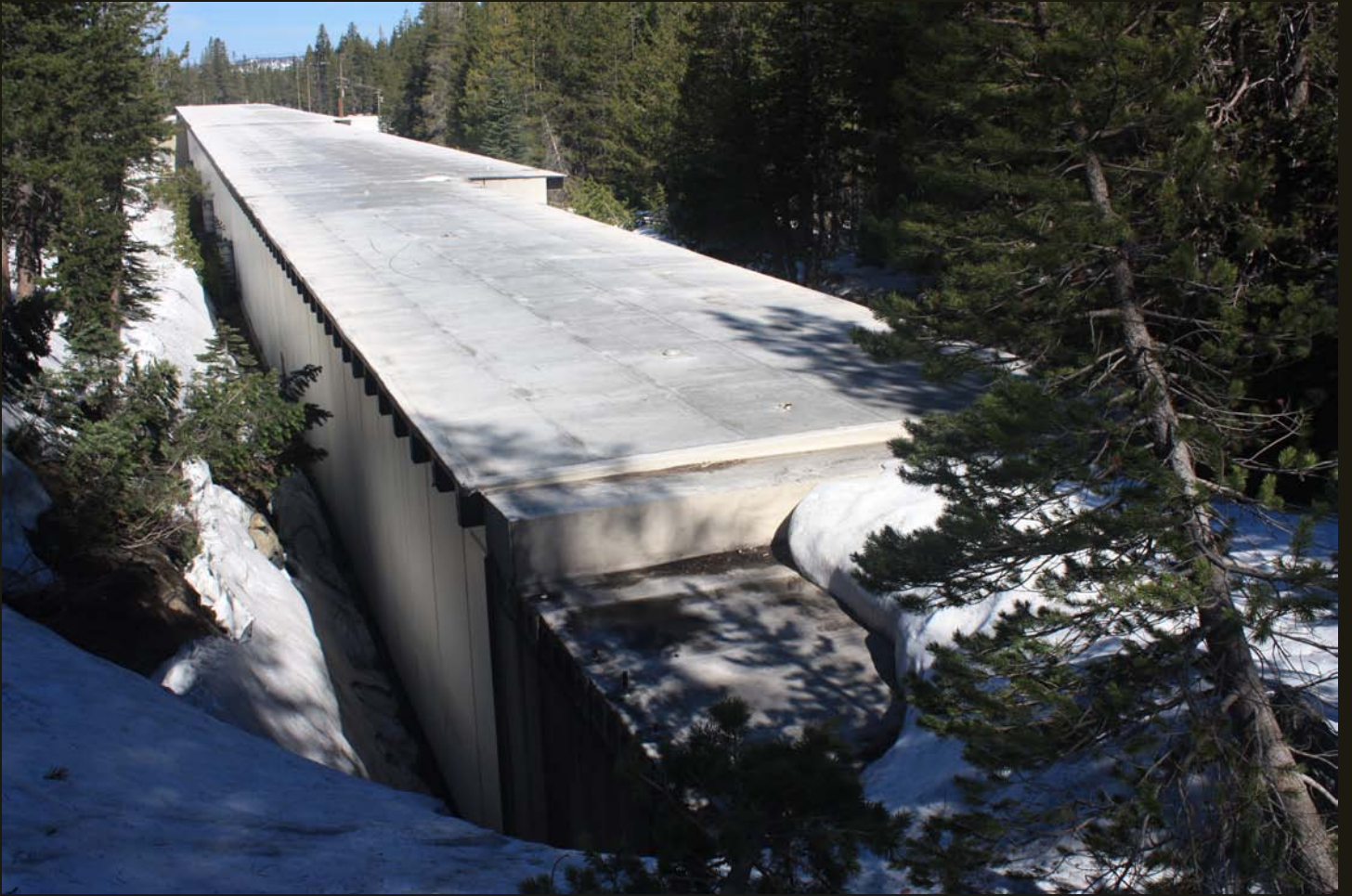
Westward view of the snowshed at the west entrance of the 1925 tunnel, which is under the snow in the foreground.
