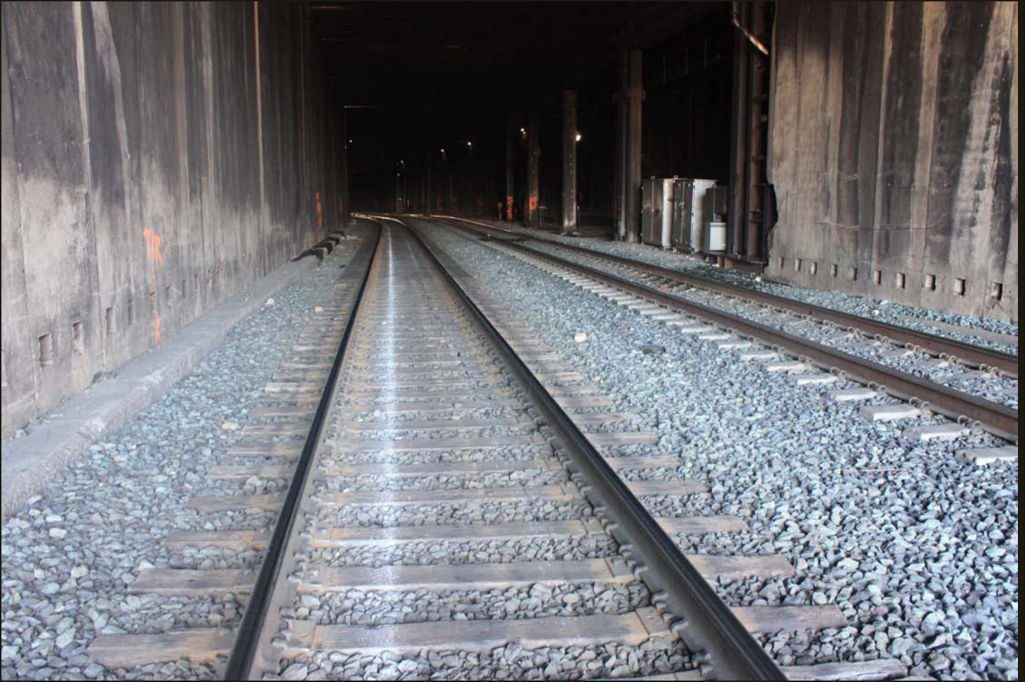
Westward view of the active shed entrance. The concrete wall on the right is the original (1925) south wall of the shed and the wall was removed to the left, where pillars replaced the wall when the wall was opened up to add the third (active entrance). The 1925 second track alignment is on the other side of the pillars and the original (1867) CP alignment is in the dark distance.
