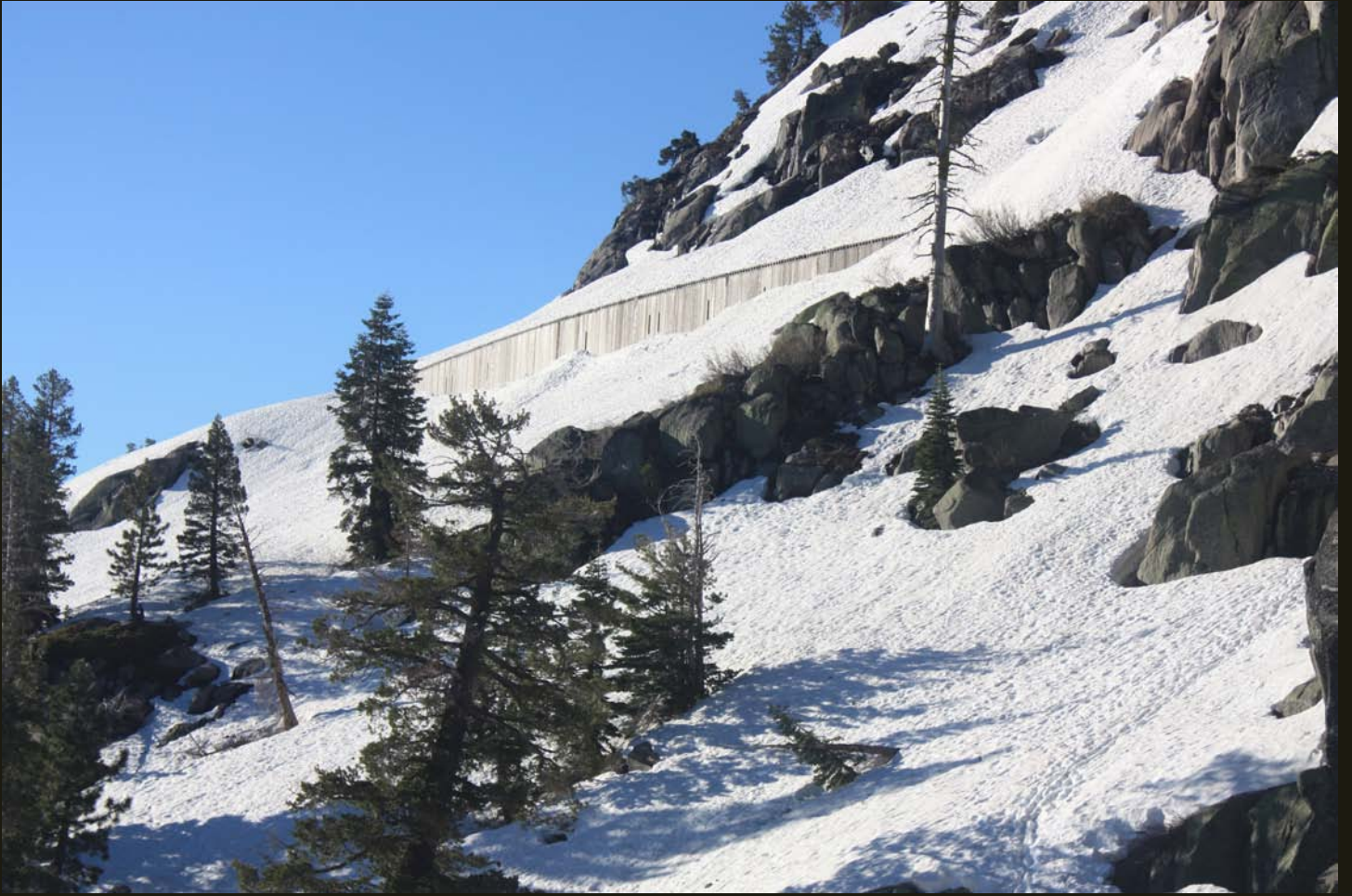
Closer view of the snowshed on the east side of the tunnel east of the China Wall.
