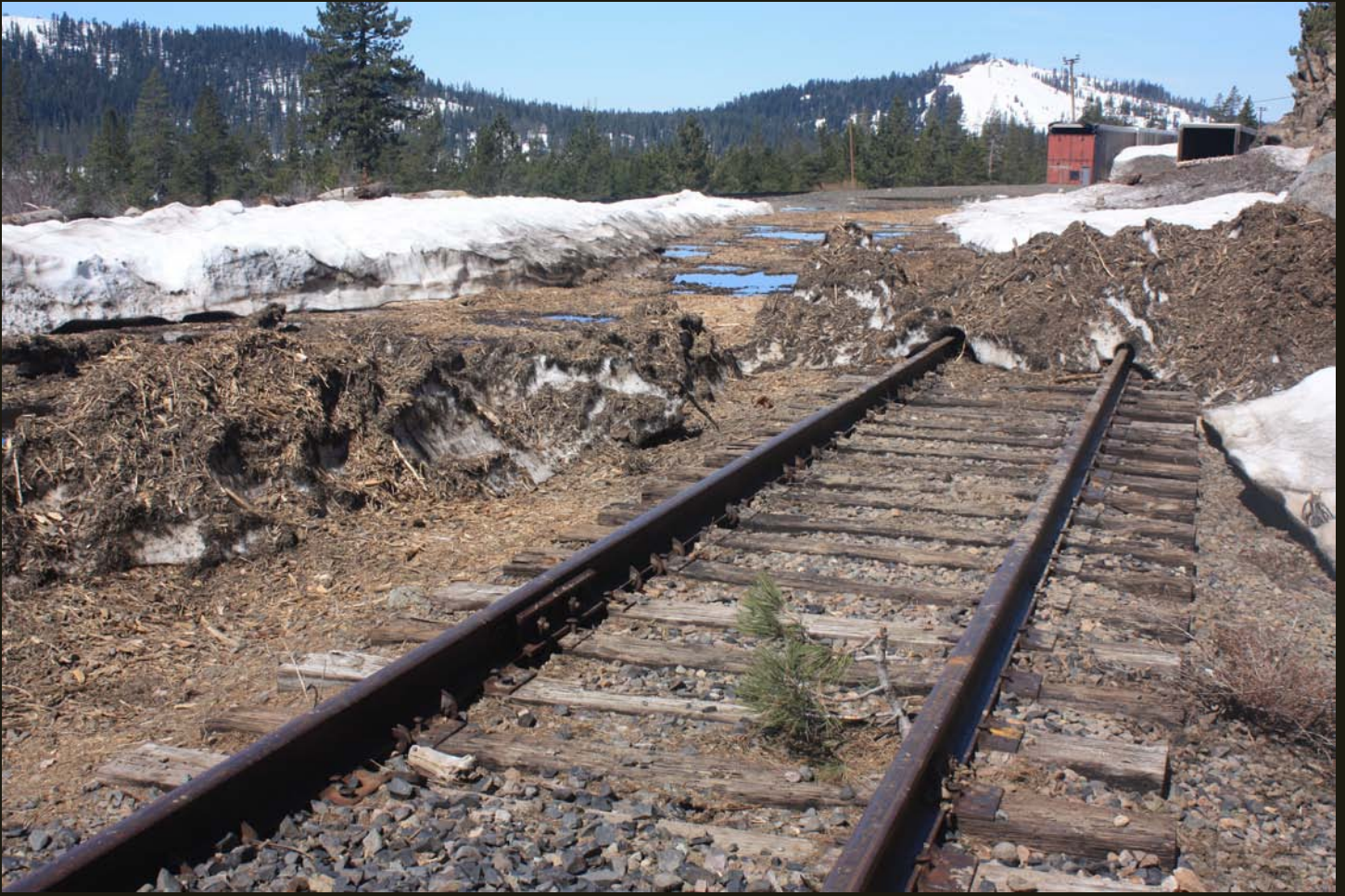
Westward view of the east entrances for the Norden snowshed complex. The original CP alignment in the foreground and still has tracks. The active track is barely visible to the left of the red door. There is a lot of snow for late May.
