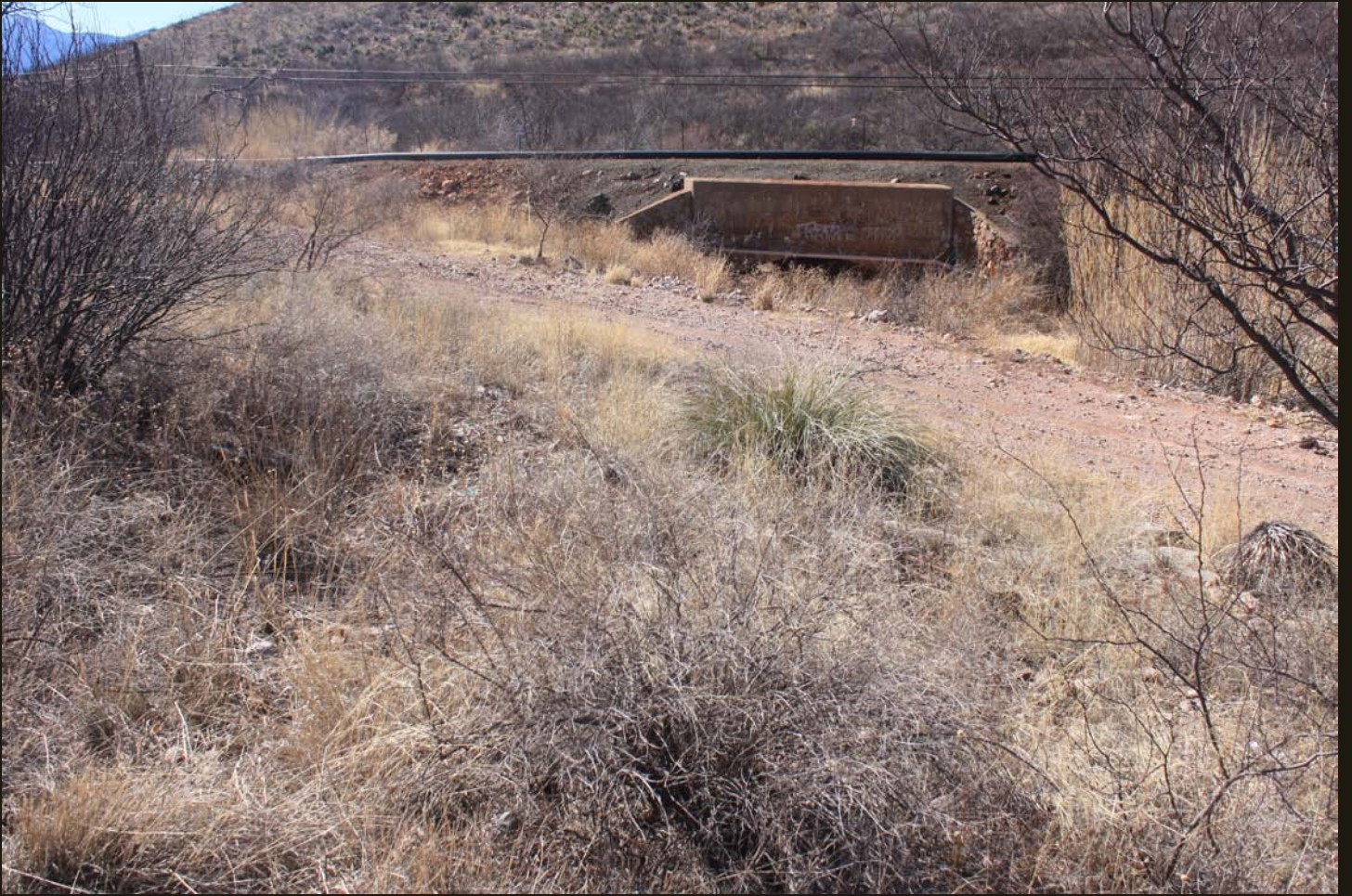
Westward view of the A&SE (1889) just south of Warren. Note the concrete culvert under the grade and the piping laid on the grade; this is the same piping seen in the first photo.
