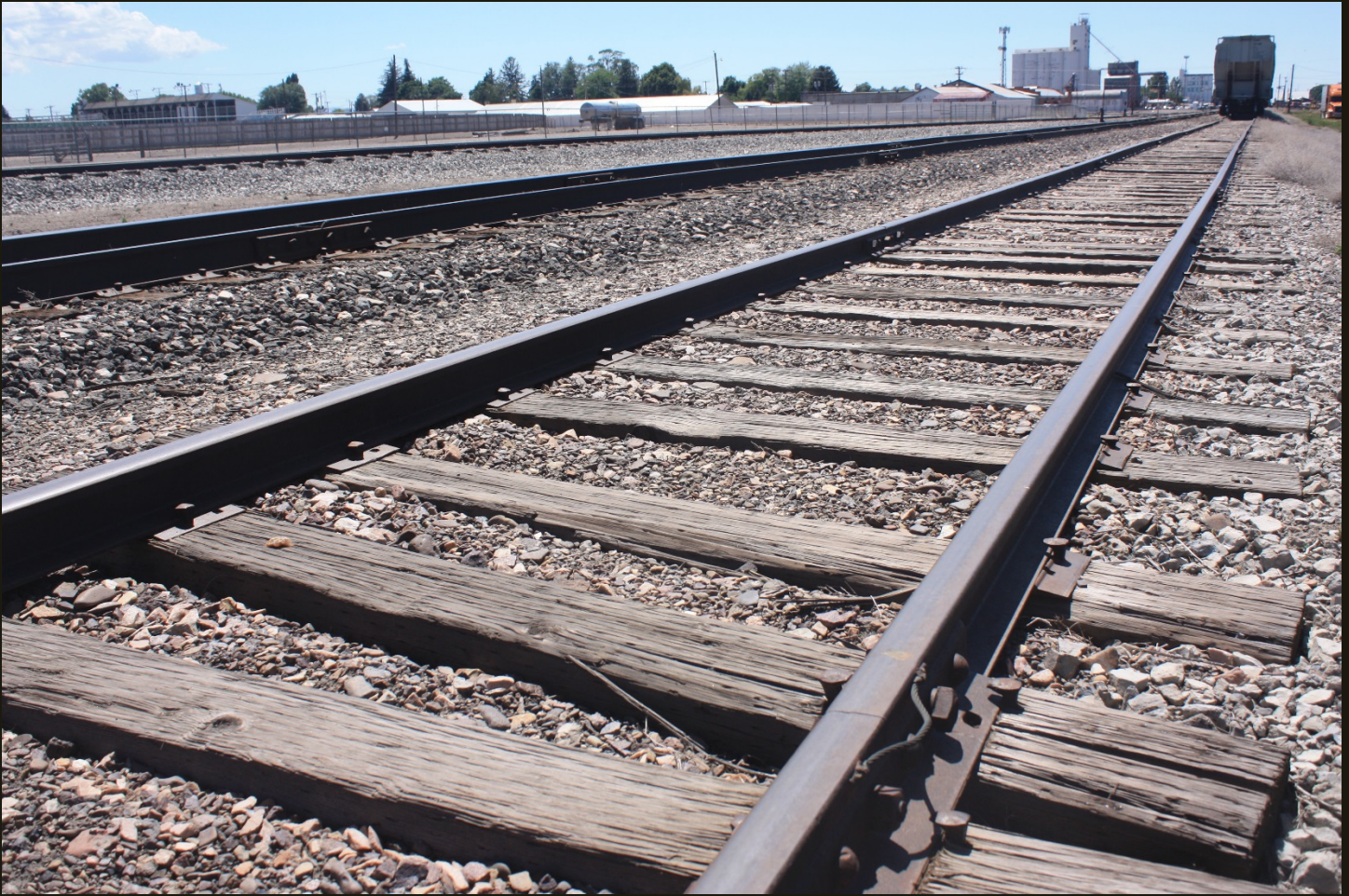
Now we've moved a mile east along the M&SW (1905) in Burley and are looking southwestward; the silos in the right distance are the same ones that are visible in the previous photo but now viewed from the other side. From right to left, the tracks are a siding with stored cars, the M&SW mainline and, to the far left, the beginning of the OSL Raft River Branch (1916).
