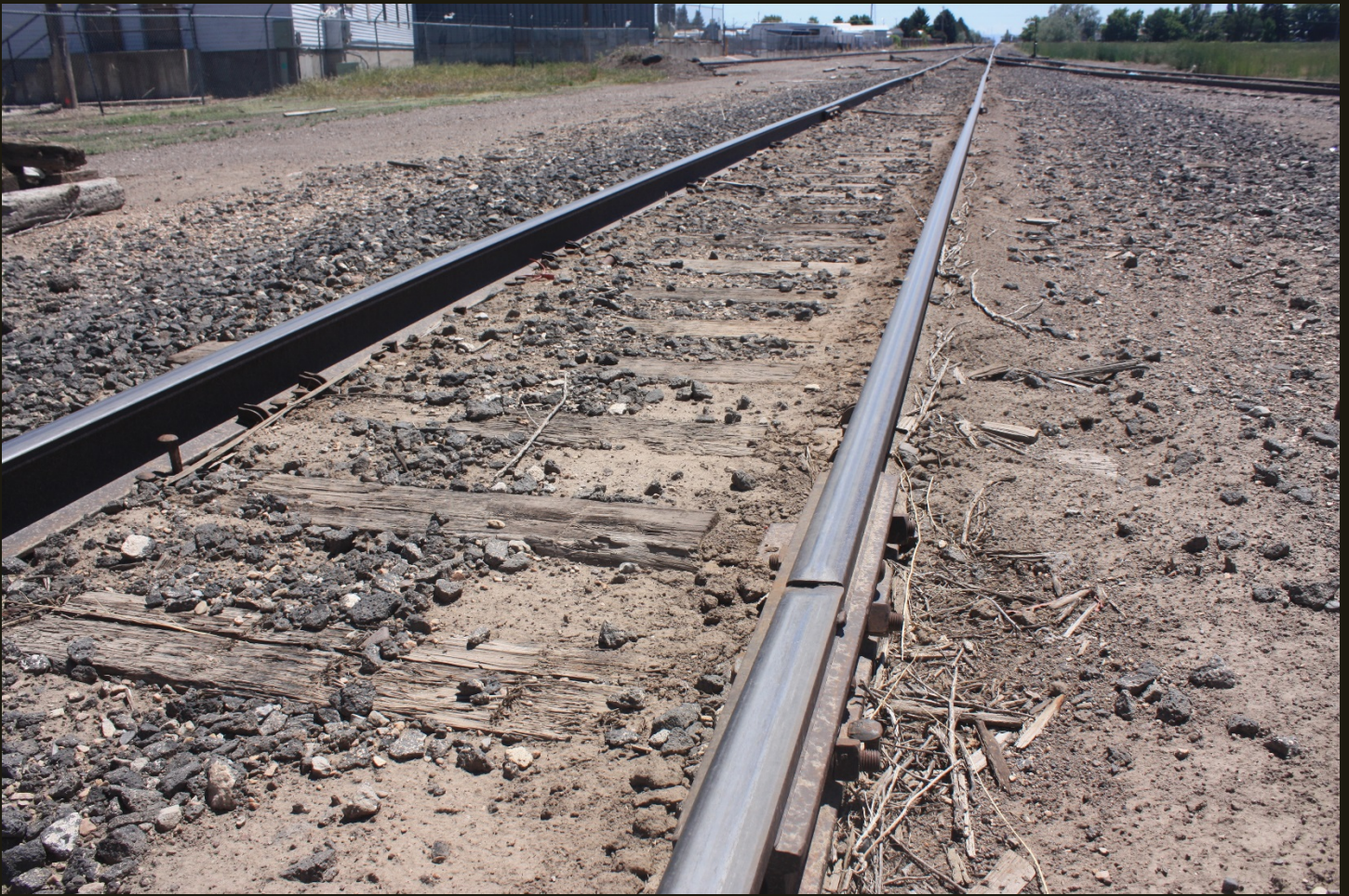
Southwestward of the OSL Goose Creek Branch (c1912), same location as previous. The switch and trackage to the right may have been the west branch of a wye but today it is cut back to a spur (see below).
