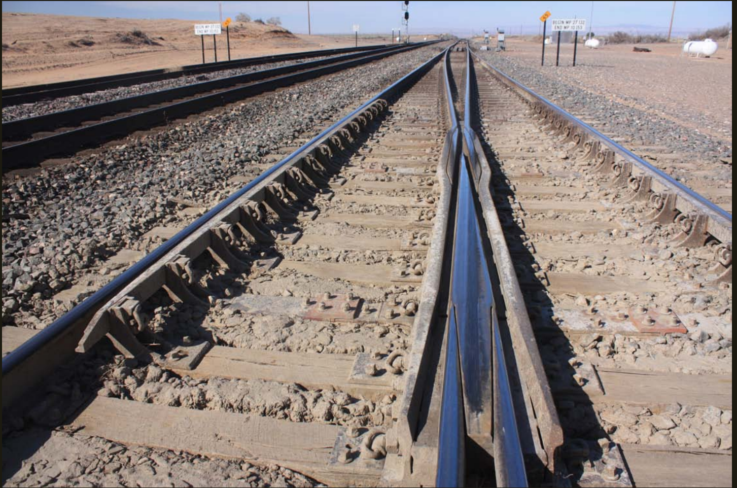
Close-up of Dalies switch, looking west.
