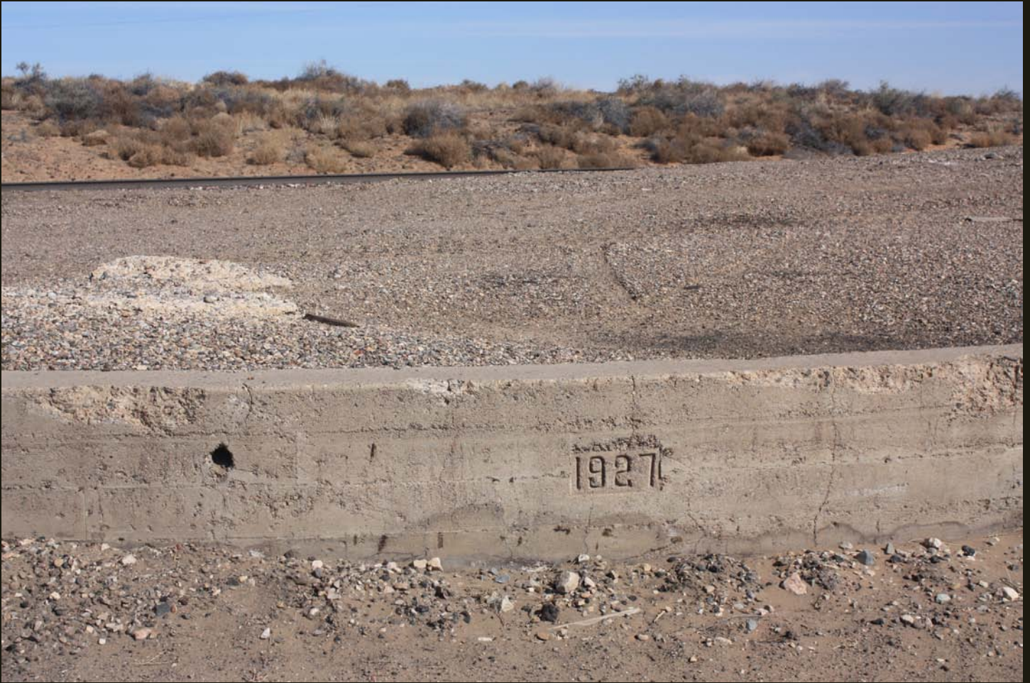
Northward view of the foundation of a 1927 loading facility along the ERNM at its western terminus at Dalies; the A&P line to Isleta is behind the foundation.
