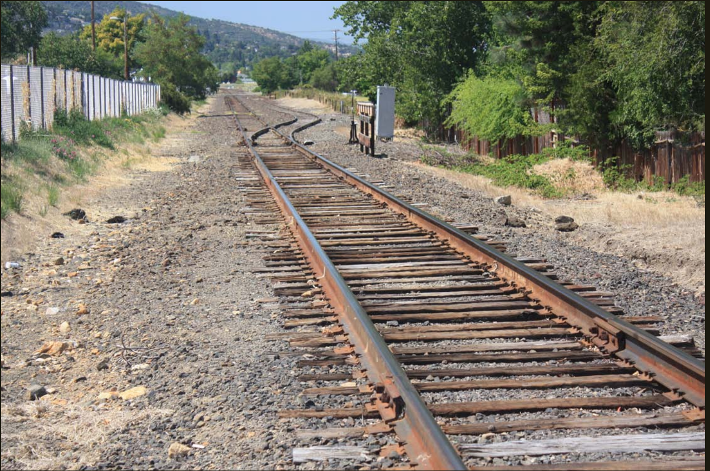
Northward view of the C&O (now CORP) line on the south side of Ashland, a few steps north of previous location; this is the first switch to the Ashland yard where, in 1887, Charles Crocker drove the C&O – O&C golden spike.
