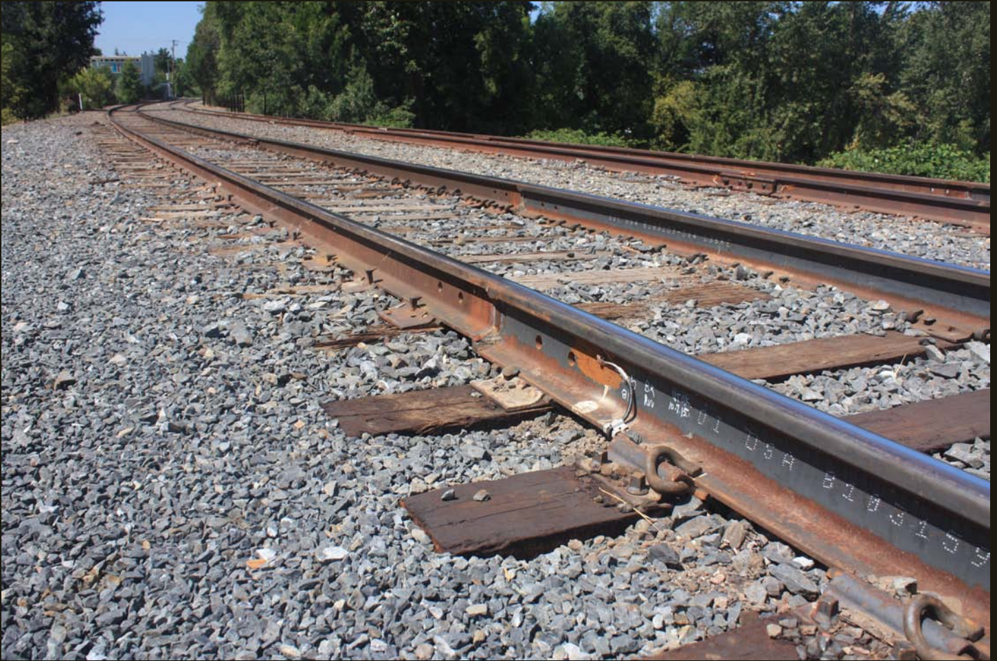
Northward view of the O&C (now CORP) line at the same location as previous. The siding continues a quarter mile farther north, then a switch takes the line back to single track. Note the welded main line track (the siding is bolted), in contrast to the bolted main line at the south end of town (first photo).
