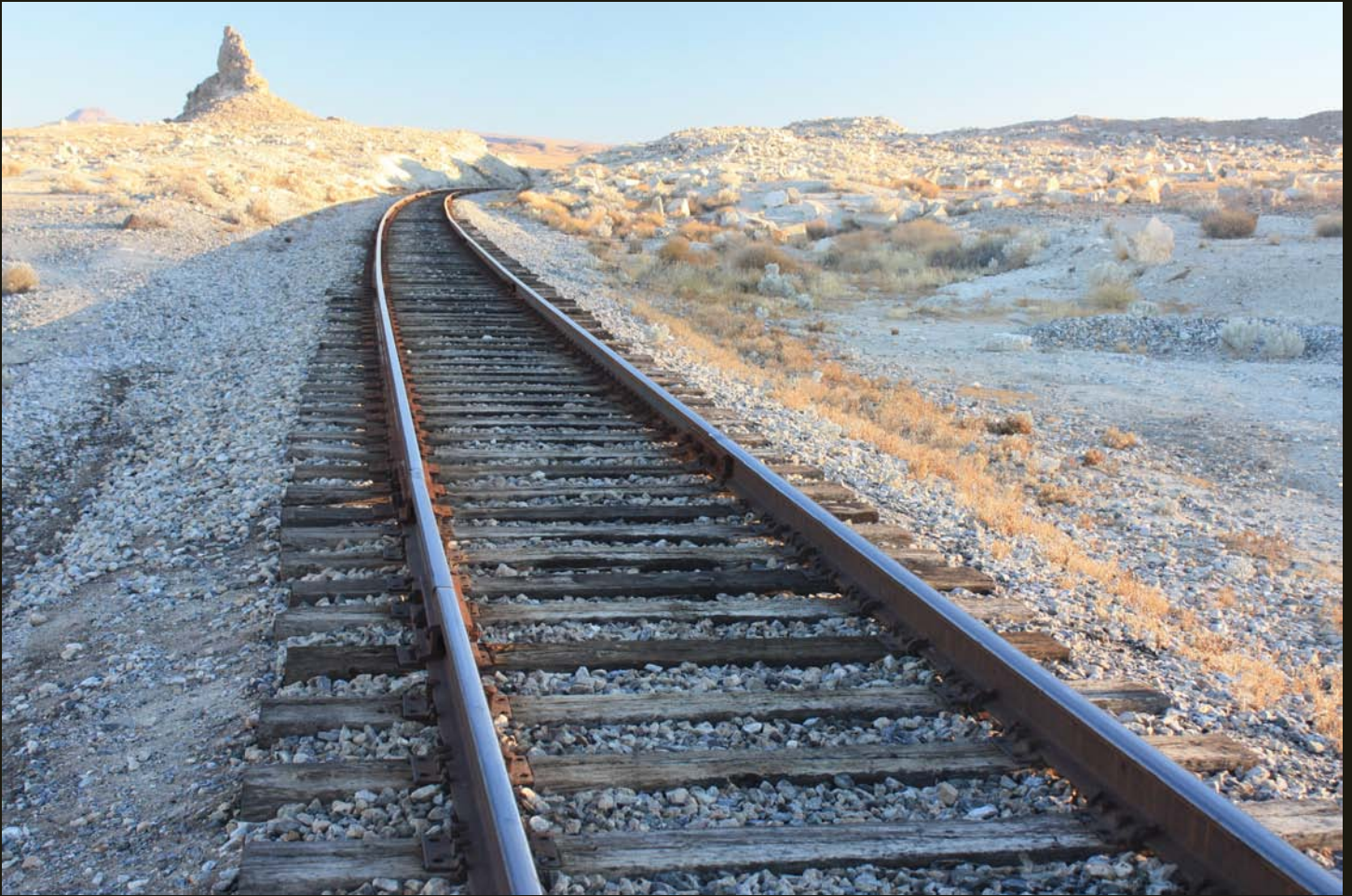
Southward view of the Trona Railway 18 miles from Searles Junction and 12 miles from the end of track at Trona. A small cut carries the grade over a low bedrock hill.
