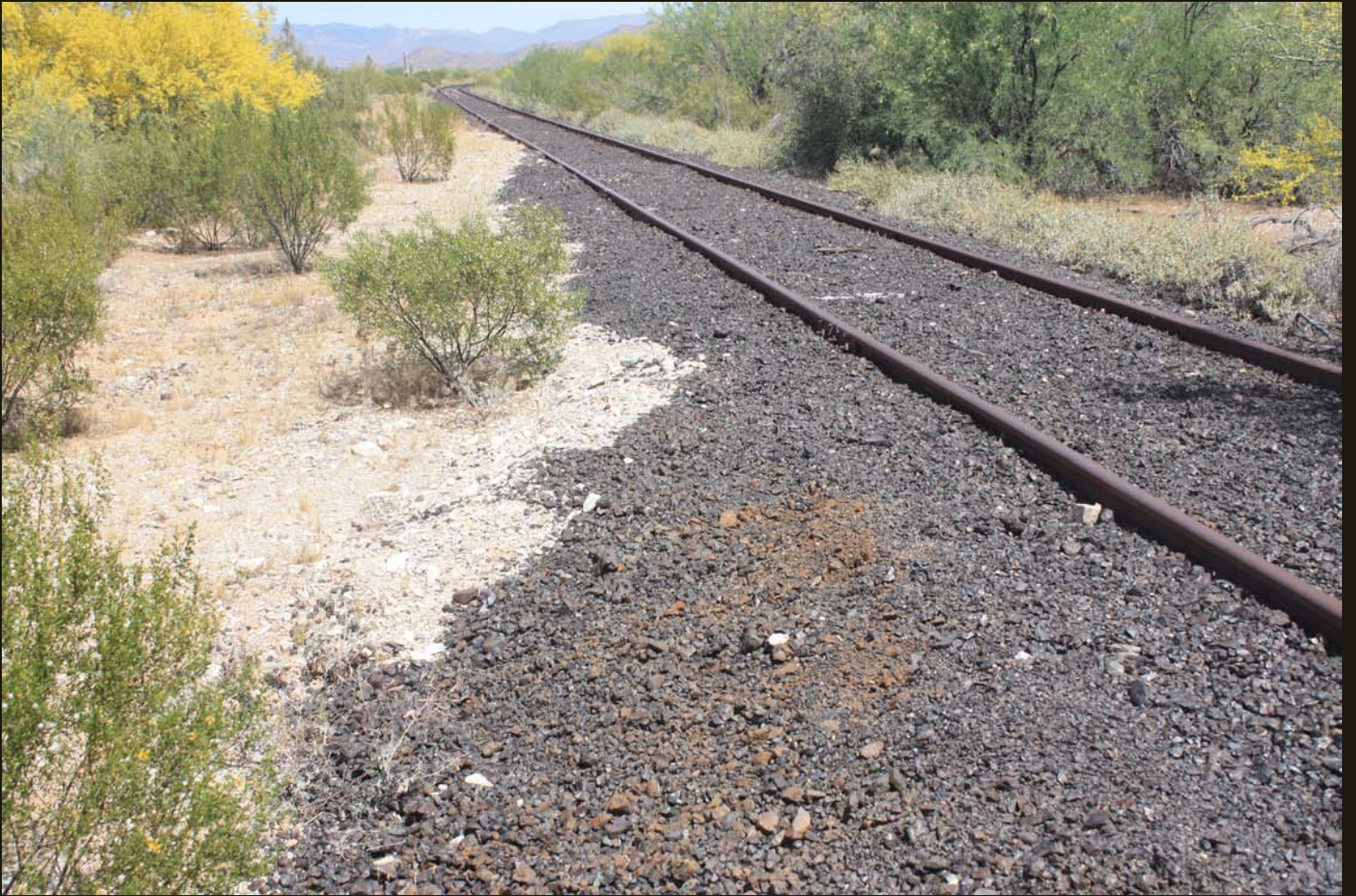
Northeast view at same location as above, where the Magma Arizona grade makes its first bend as it enters the Pinal Mountains toward Superior.
