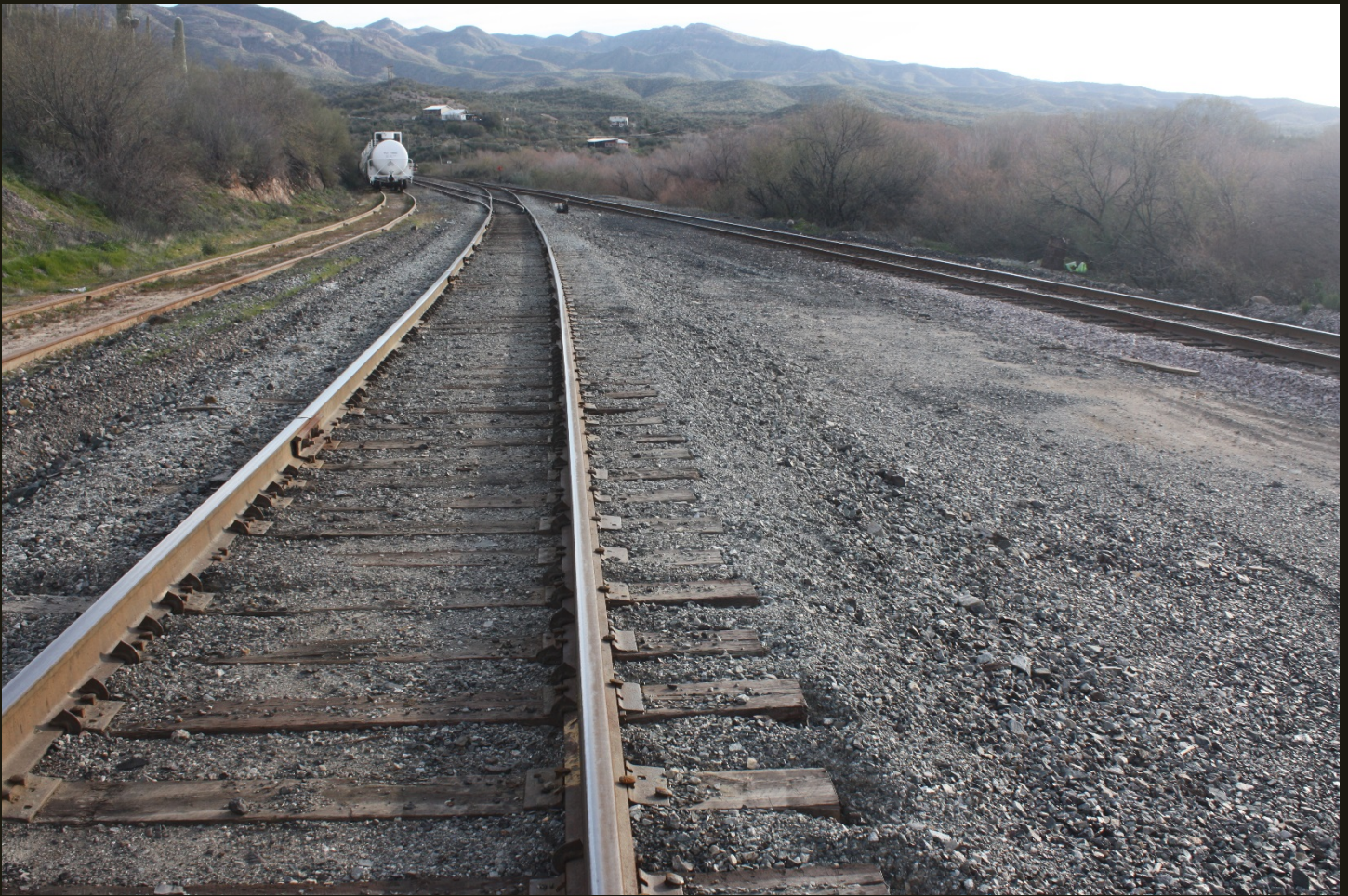
Eastward view, same location as previous. The tracks are, from left to right, a siding for the R&GV (with stored tank cars), the R&GV mainline (foreground), and the P&E (1904) mainline. The R&GV and the P&E (1904) join at a switch in the distance – that switch is Ray Junction – just beyond a closer switch that splits off another siding of the R&GV before joining the P&E (1904).
