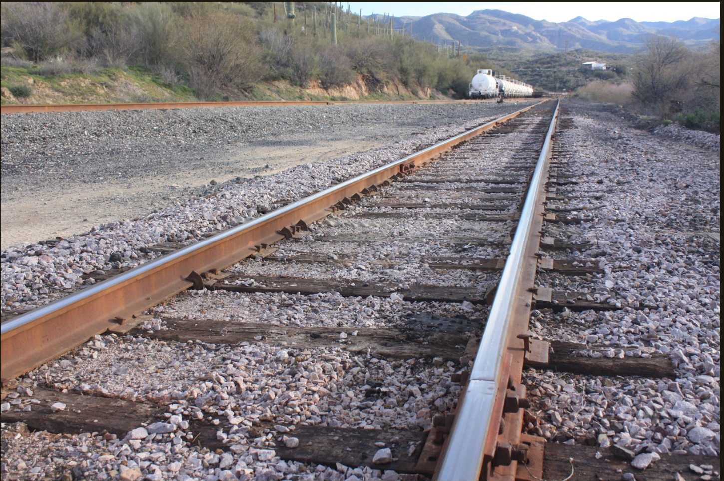
Eastward view a few steps south of previous location. The P&E (1904) is in the foreground and joins the R&GV in the distance. Note the iconic saguaro cacti above and to the left of the stored tank cars.
