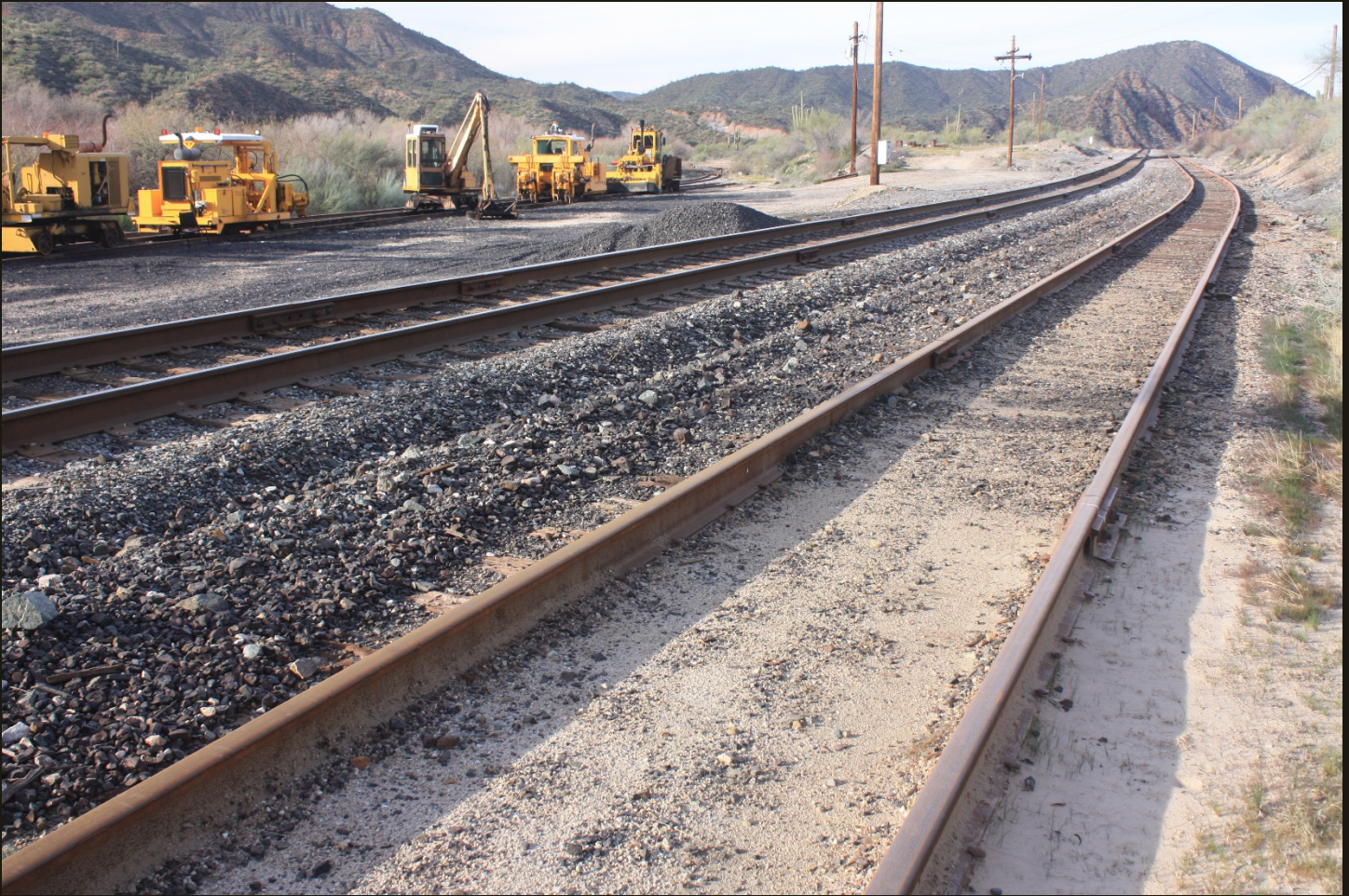
Westward view a few steps north of the previous location, with the same yellow iron maintenance equipment on a siding. The tracks are, from right to left, a siding for the R&GV, the R&GV mainline, the P&E (1904) siding (with the yellow iron), and (barely visible) the P&E (1904) mainline. This part of the R&GV, including the almost one mile of track between Ray Junction (this location) and Kelvin, was built in 1910 and is not on the RMC (1899n) alignment.
