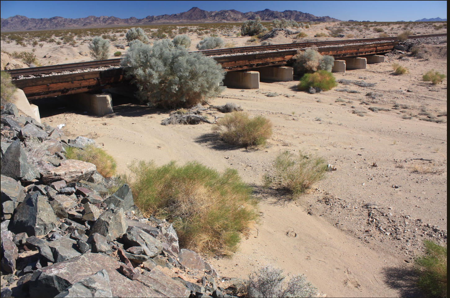
A low bridge carries the A&C (1910) over a wash at same location as previous.
