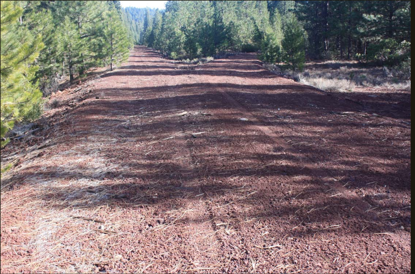
Eastward view of the western branch of the Bartle wye, where the MR arrived in 1905.
