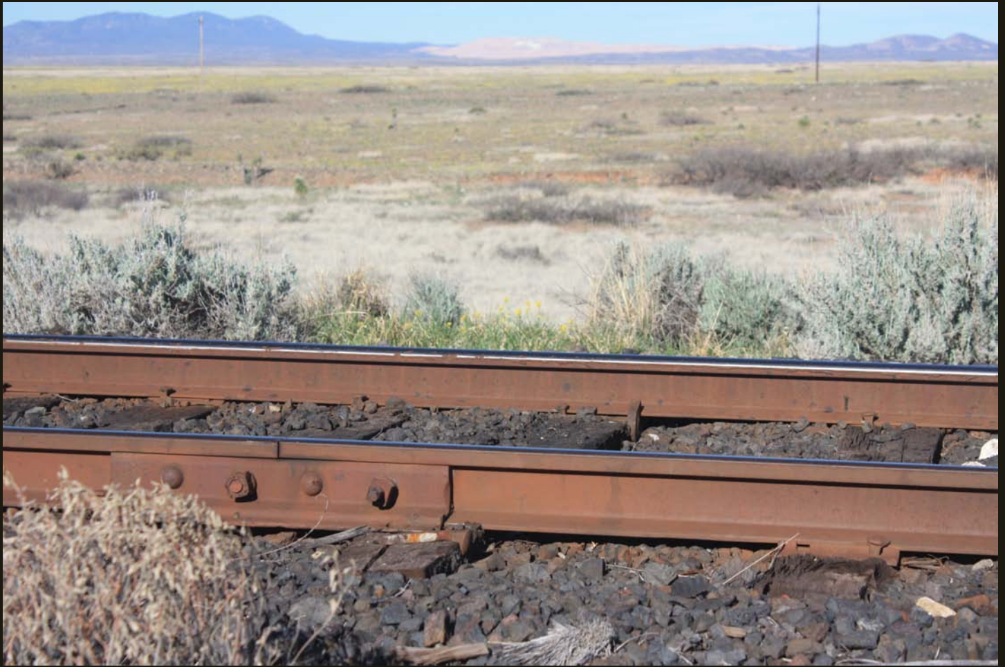
Westward view of the SC&N a few miles south of Hurley, with the Phelps Dodge open-pit copper mine at Tyrone in the background, at the Burro Mountain Railroad end-of-track. The low ridge at the Tyrone mine is the continental divide.
