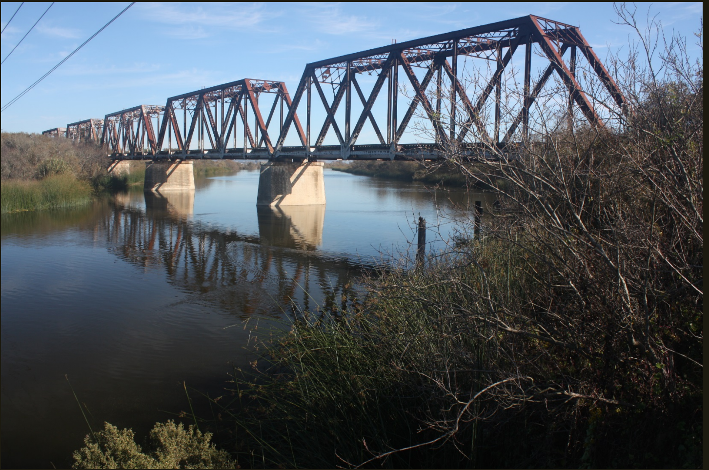
Three miles southwest of the previous location looking eastward at the bridge that carries the SP Monterey Branch (1879) over the Salinas River.
