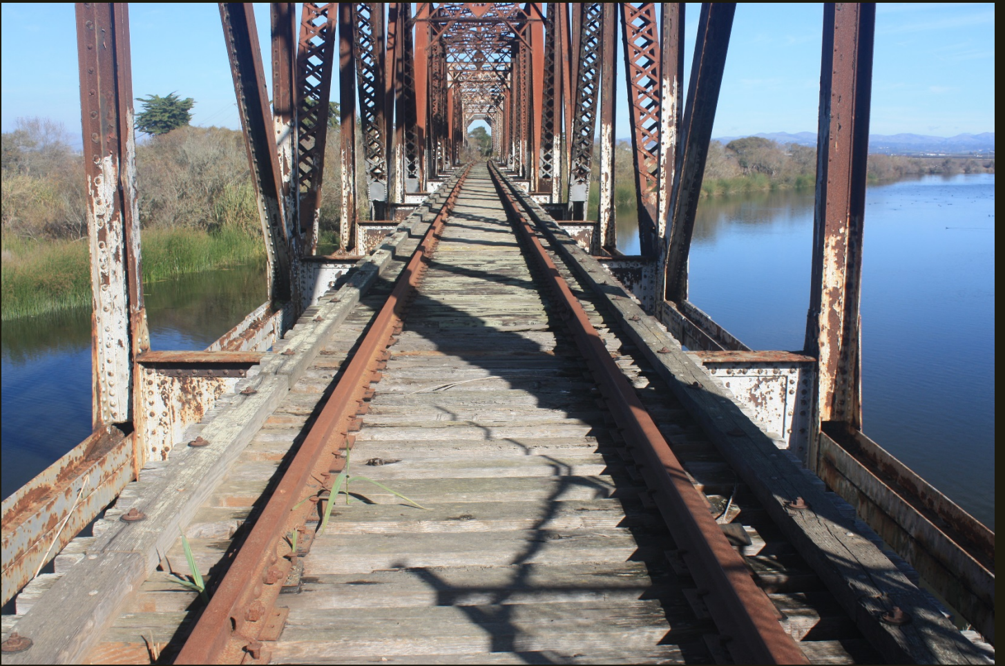
Northeastward view of the bridge that carries the SP Monterey Branch (1879) over the Salinas River.
