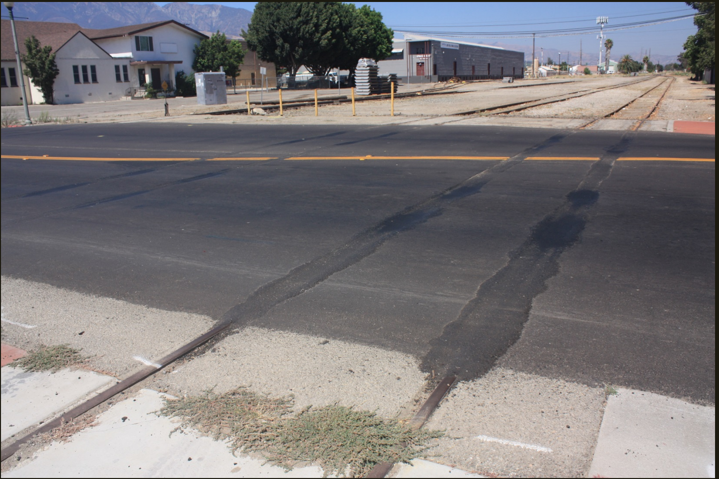
Eastward view of the SP Santa Barbara Branch (1887) Santa Paula railyard, just east of the depot (shown in the first photo). In 2018, when this photo was taken, the tracks were covered with asphalt patch, so F&W trains from Fillmore cannot cross the street (10 th Street) to the depot. I don't know if the patch has since been removed.
