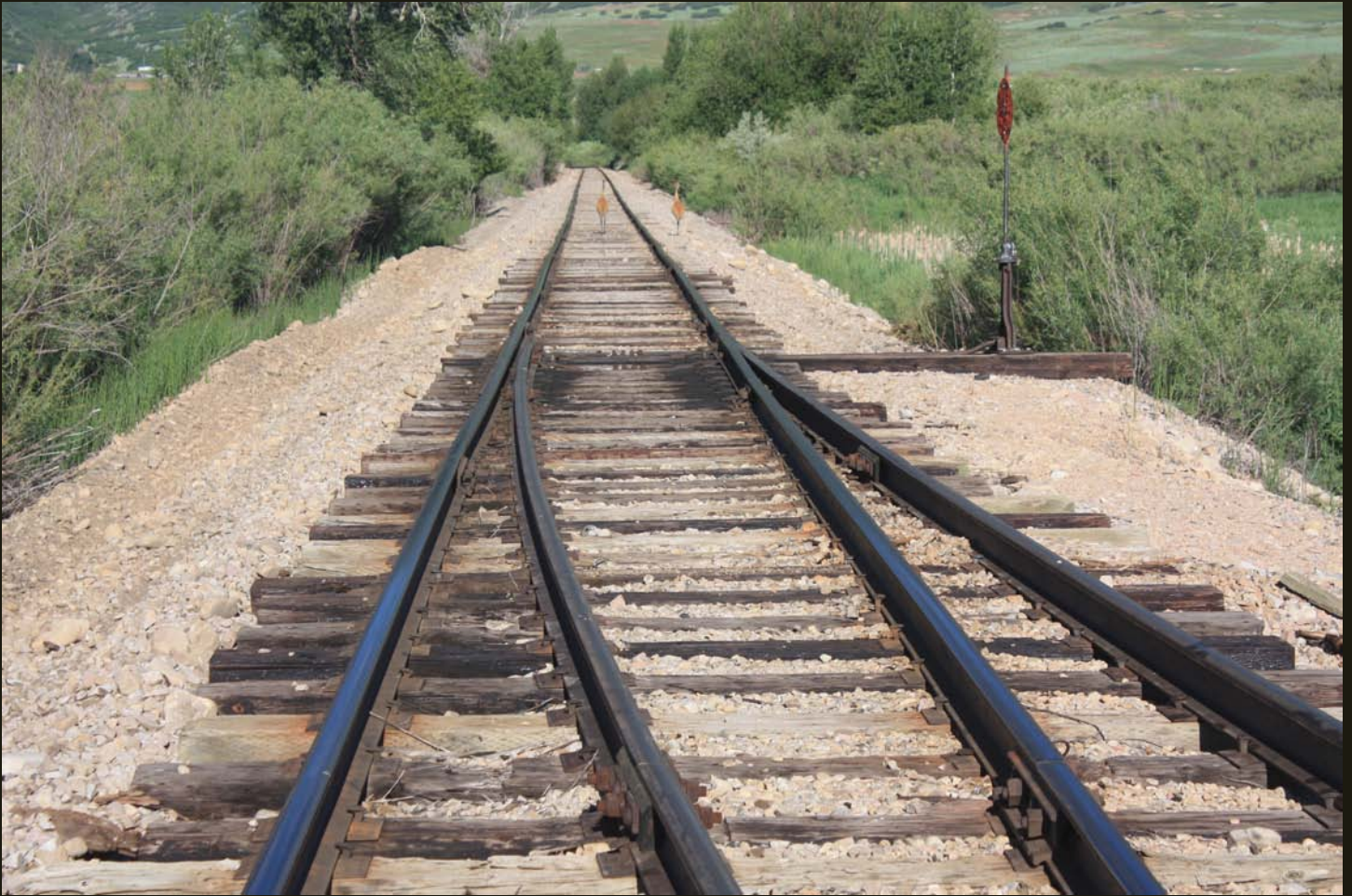
The switch in the foreground is at the far end of the HV siding in the previous photo. On this June day in 2015, two Sandhill Cranes ponder the 1899-vintage railroad.
