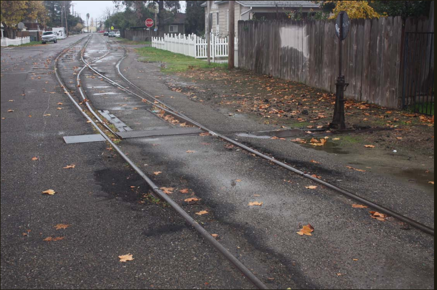
Eastward view of the same switch as in the previous photo. A non-residential building at the end of the street is the beginning of the old industrial TS end-of-track in Turlock.
