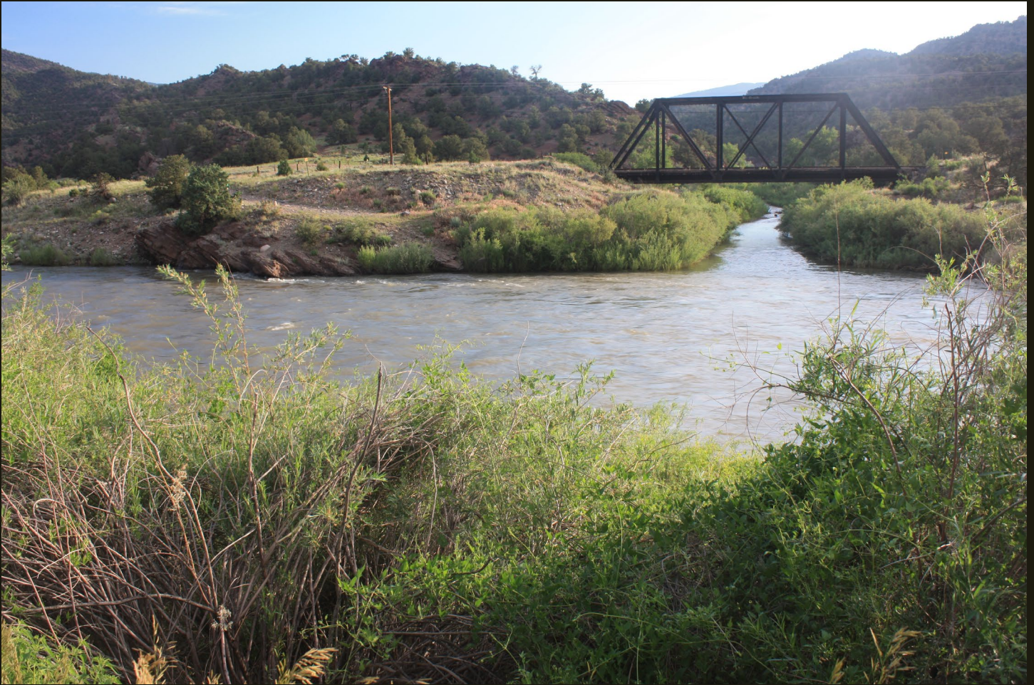
Northward view of the D&RG Leadville Branch (1889n) 10 miles southeast of Salida on the Arkansas River. The bridge that carries the tracks across a tributary of the Arkansas River may have been built when the line was standard gauged around 1890.
