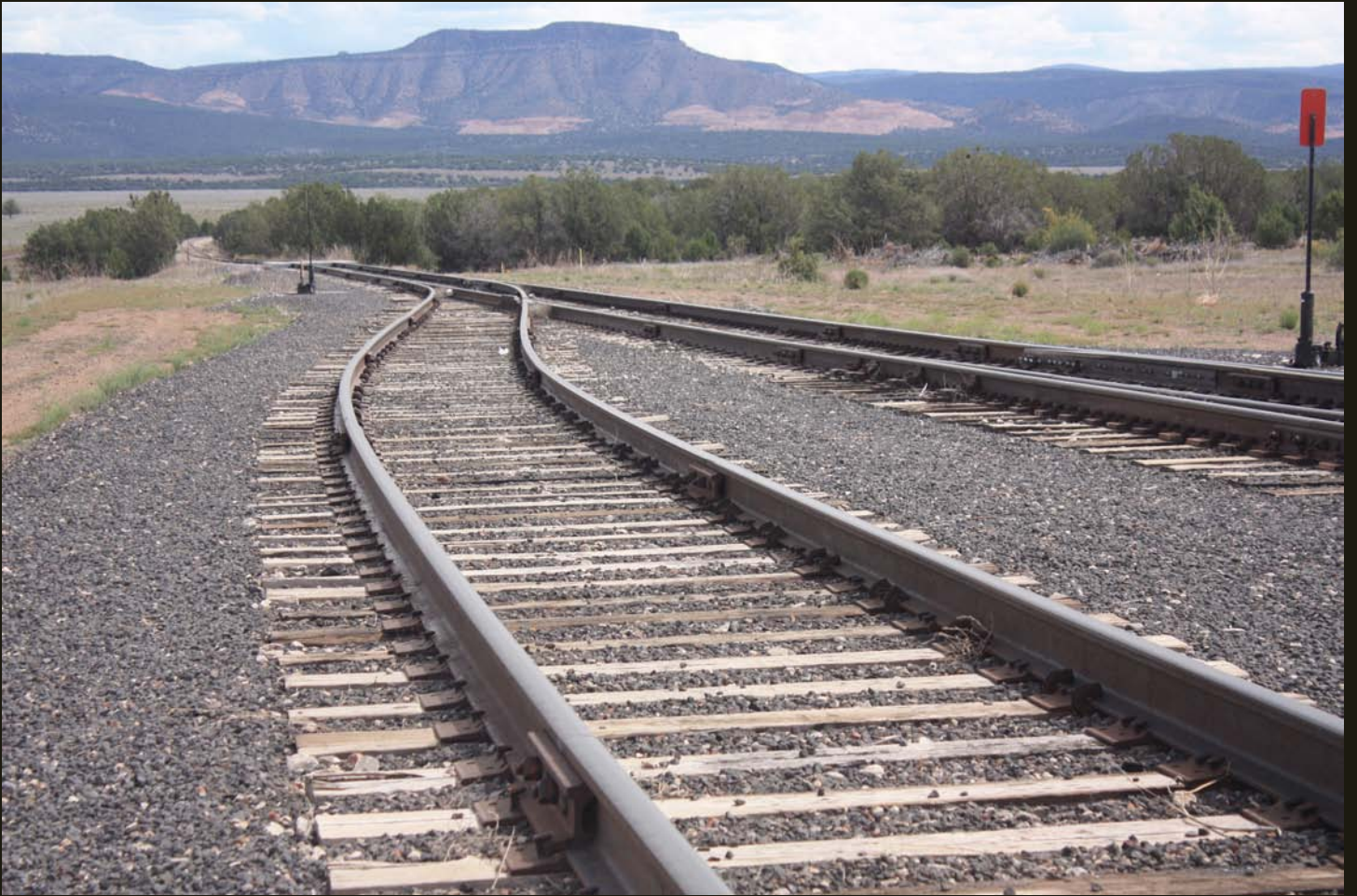
Eastward view of the VV, 500 feet east of previous location, where sidings finally converge to one track. Note bolted rails.
