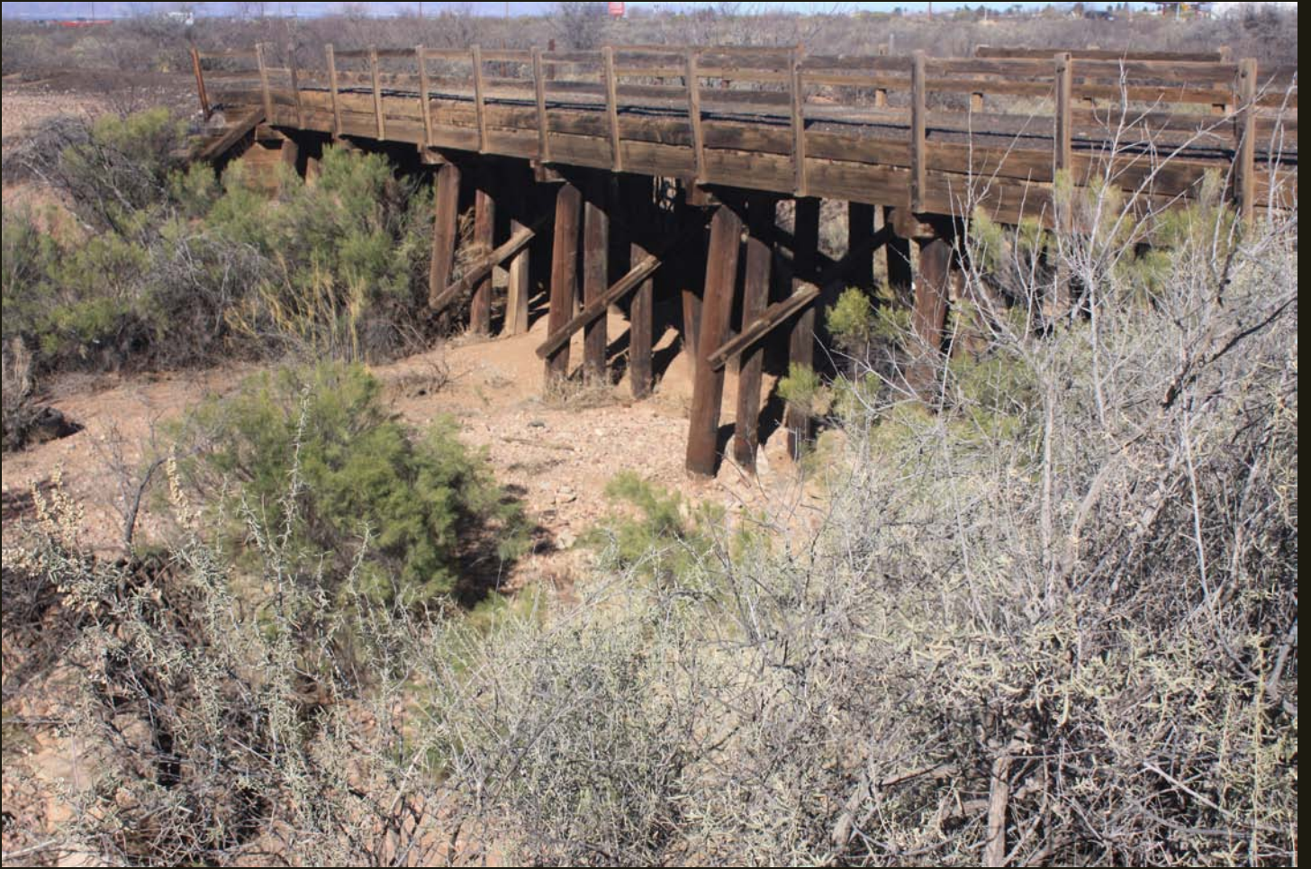
Another view of the EP&SW trestle over a tributary of Whitewater Draw at the west end of the Douglas yard.
