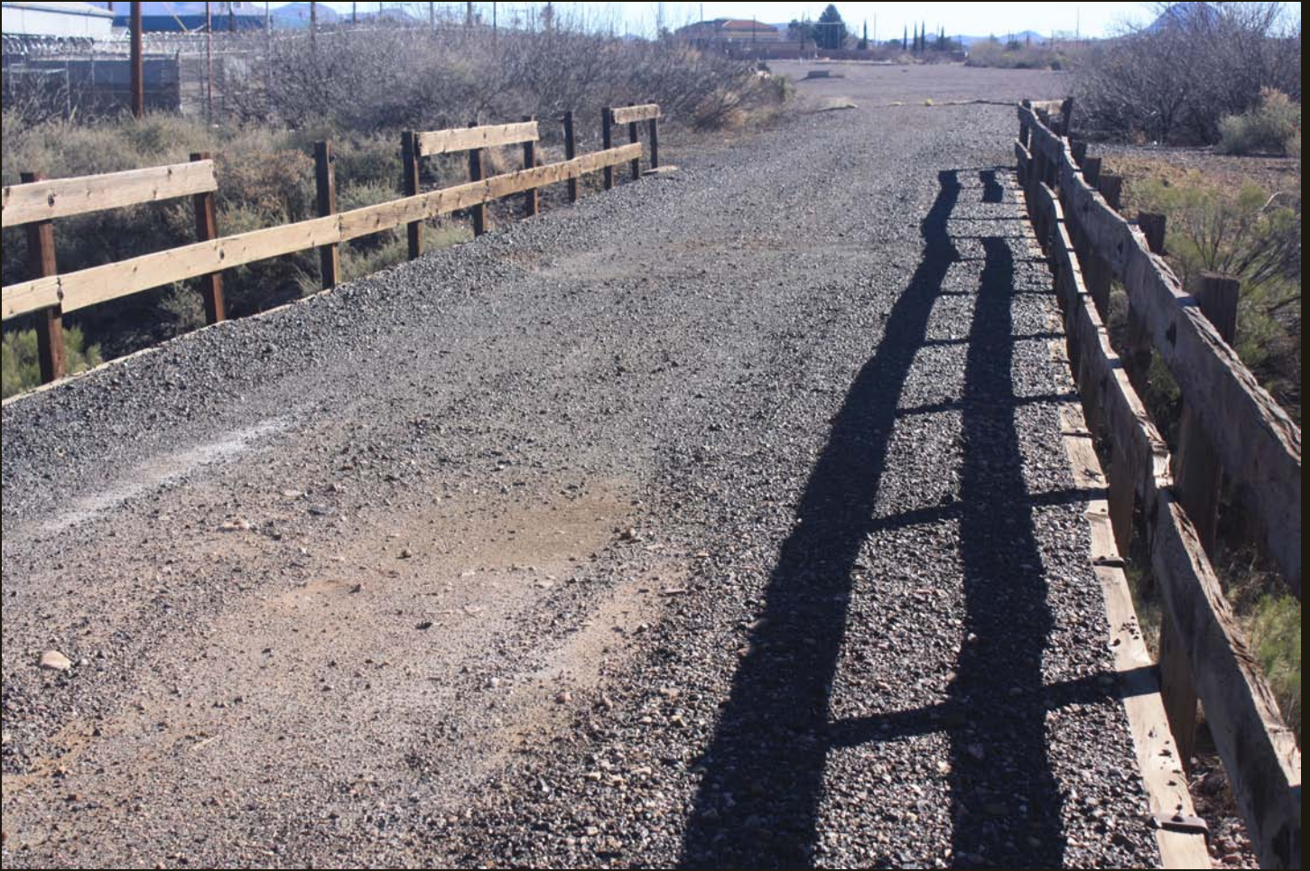
Eastward view of the EP&SW trestle at the west end of the Douglas yard. Note that the black ballast widens just beyond the trestle to what was once the Douglas rail yard. The masonry building in the center distance is the EP&SW's Douglas Depot.
