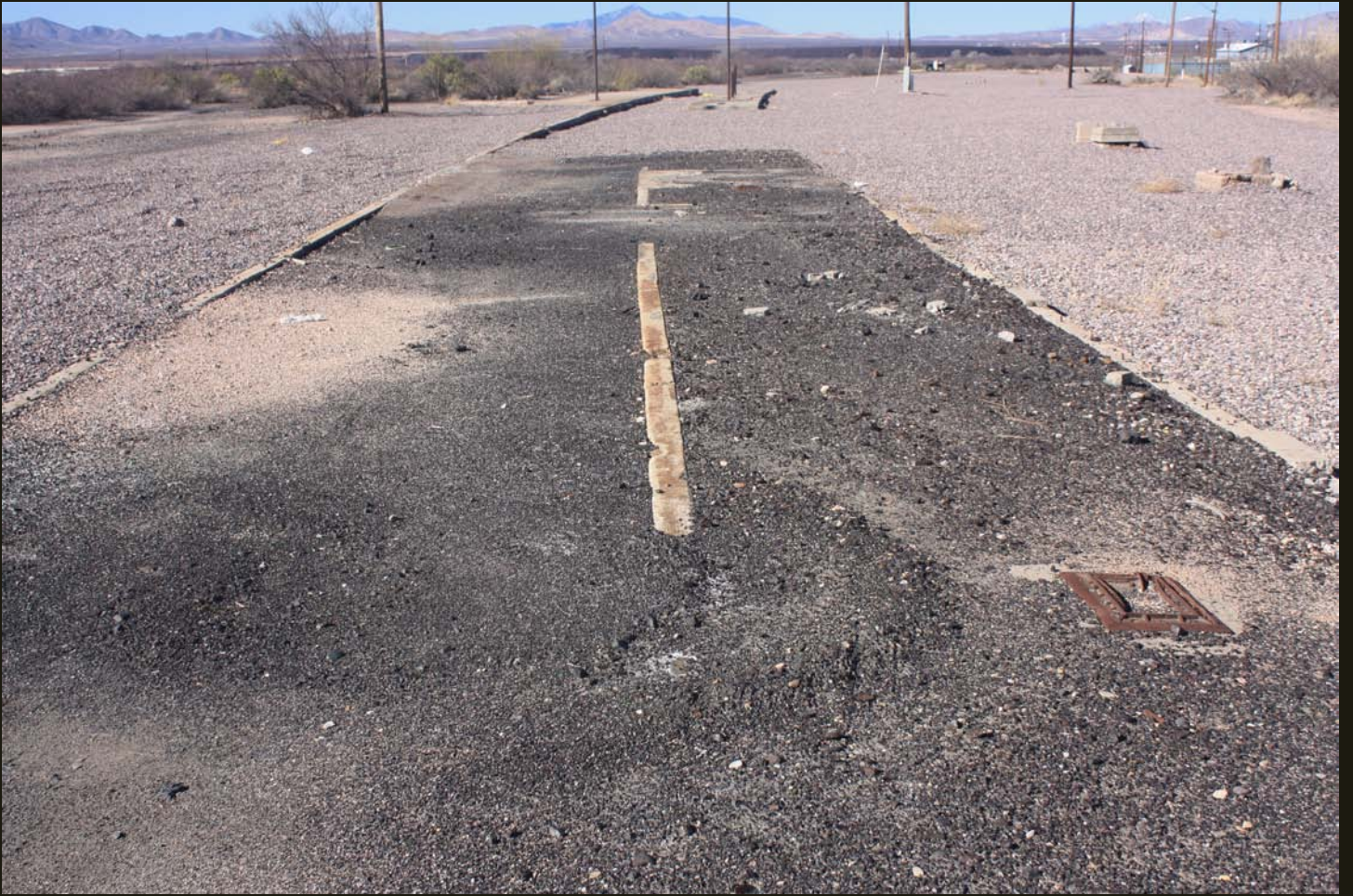
Southwestward view of old foundations in the EP&SW (1902) Douglas yard. The size of the slag pile can be appreciated in this view.
