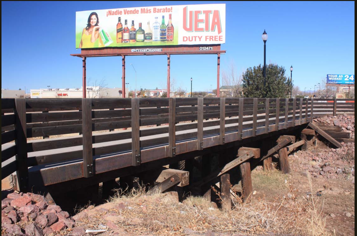
Northwestward view of a small trestle for the abandoned Nacozari (1902) a mile south of the Douglas Depot. The grade is now a rail-to-trail that connects the Douglas Depot with the Mexican border, which is 1,000 feet farther south.
