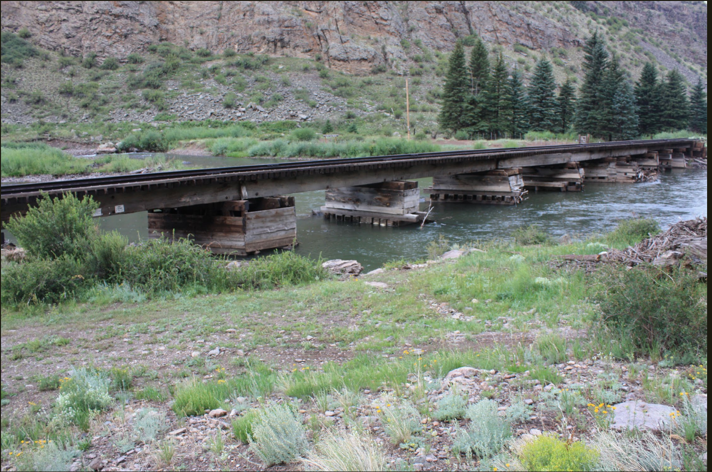
Westward view of the bridge across the Rio Grande at Wagon Wheel Gap; it is apparent in this view that the bridge is made of stacked rail ties.
