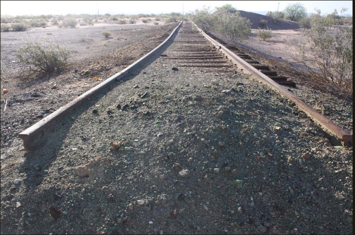
Southwestward view of the end of the turning wye, which is much longer than it would need to be to turn an engine and tender. The length of the wye and the berm to the right of the track suggest that the wye was used for loading.
