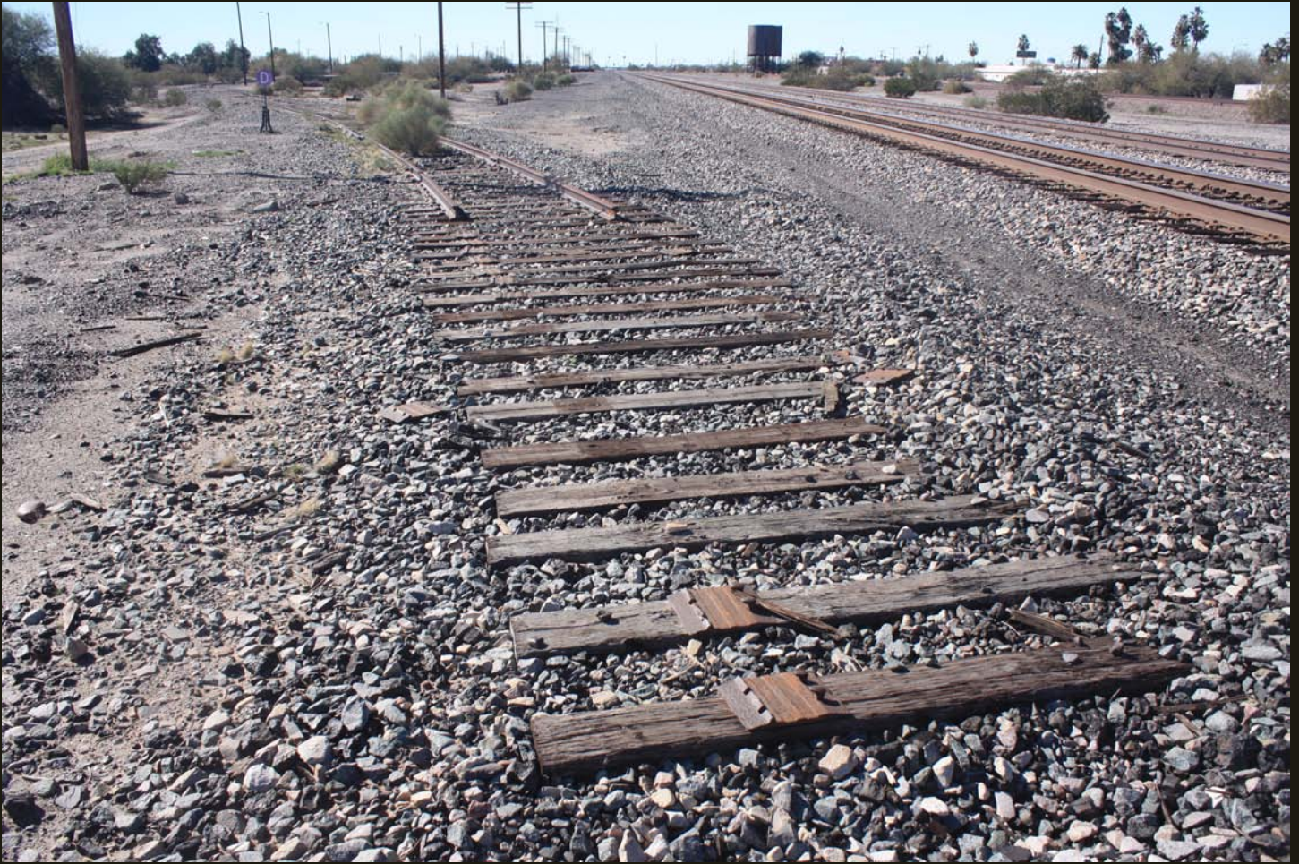
Eastward view at same location as previous. The TC&GB is in the foreground, with some rails removed, the SP (1881) double track mainline is to the right, and the two SP sidings and water tower are at the far right distance.
