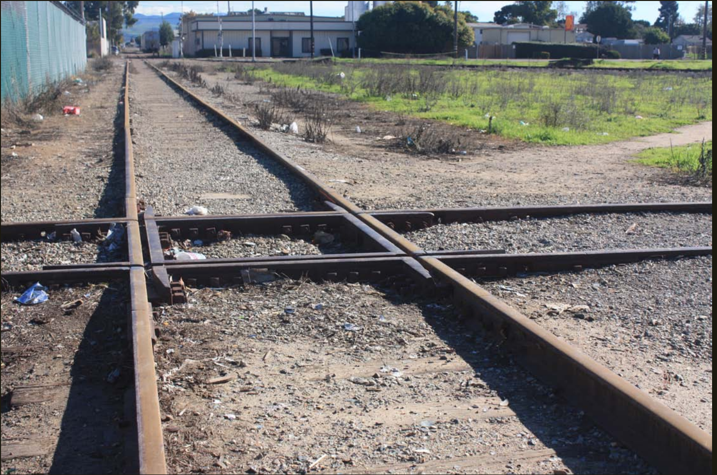
Now we are back at the crossing between the SLO&SMV (1882)/PC (1887) and the SMV (1911) looking east toward Gates and Roadamite. The SMV track has been cut back to a point half mile down the line (east) from this crossing.
