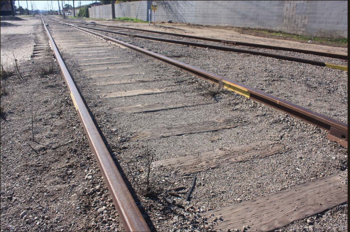
Southward view of the PC (1887) grade, same location as the previous photo, with the western half of the SMV (1911) wye merging onto the grade from the right.
