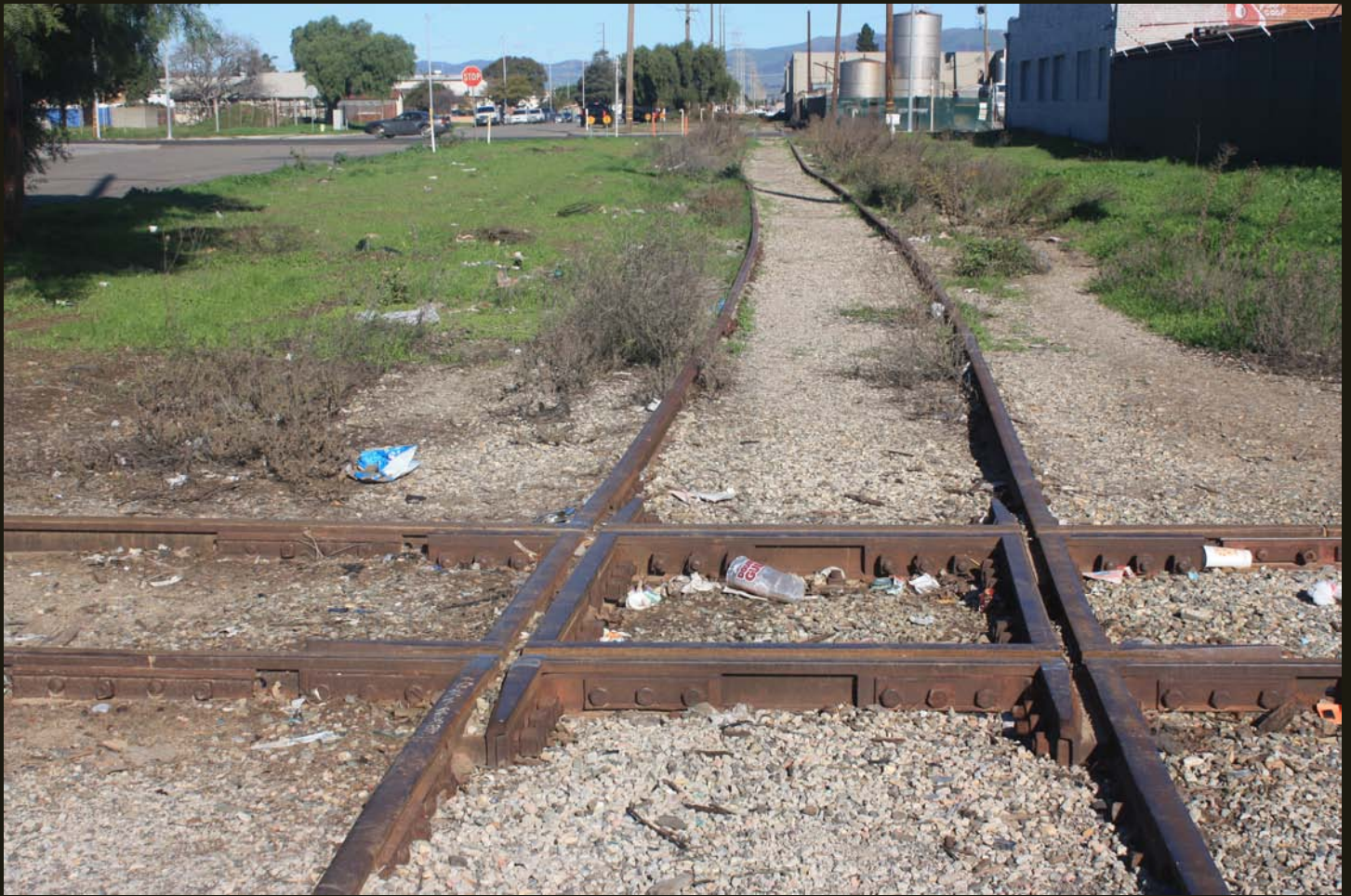
Northward view of the SLO&SMV (1882)/PC (1887) grade, 800 feet south of the previous location, where it crosses the SMV grade in Santa Maria. This location is near the SLO&SMV (1882) end of track, where the first narrow gauge construction under the PC moniker commence southward, ultimately to Los Olivos in 1887.
