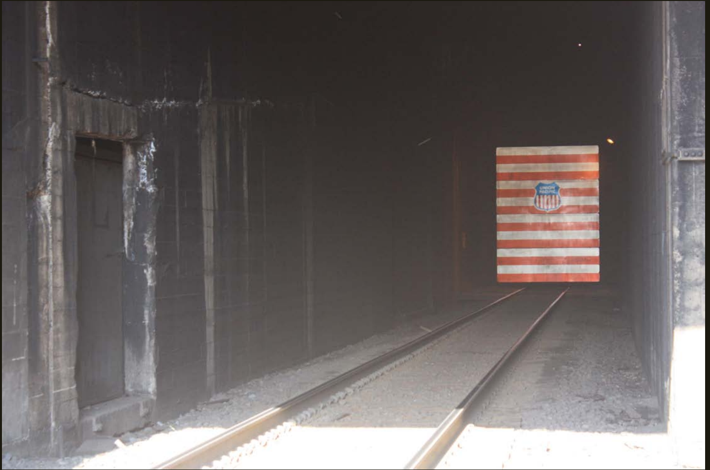
The East Portal of the Moffat Tunnel. I don't know what the UP tarp is for.
