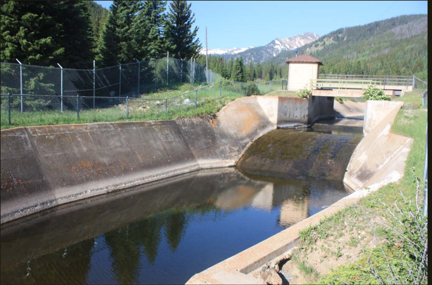
Water flows out of the Moffat Water Tunnel and adds to the flow of Boulder Creek for downstream use.
