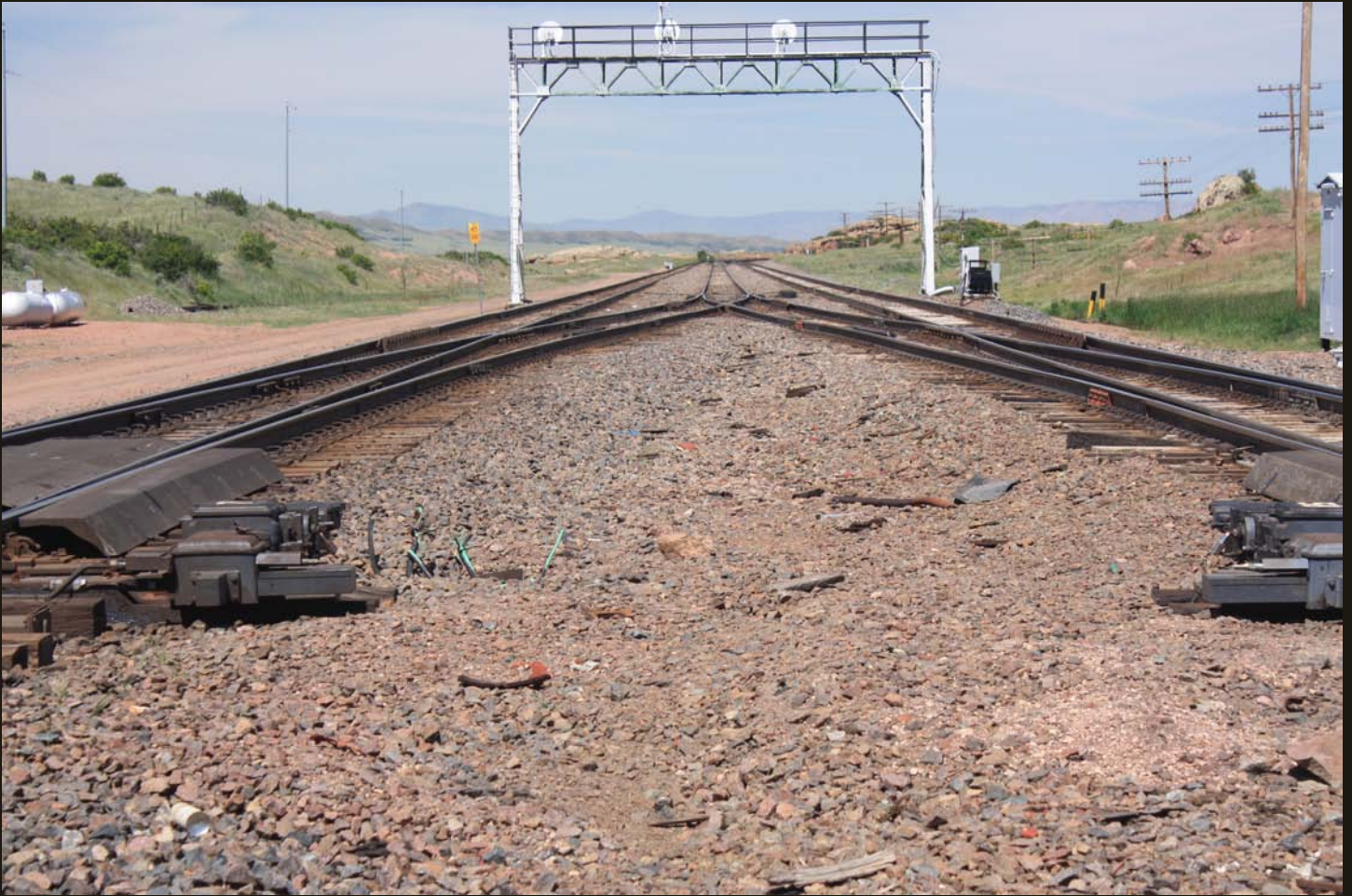
Eastward close-up view of the addition of a third track east the Hermosa Tunnel.
