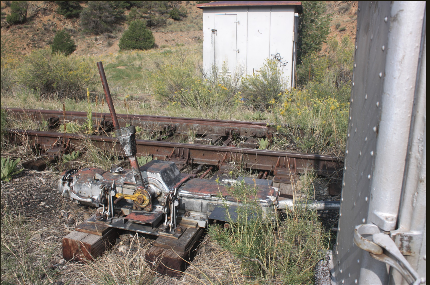
Detail of the switch for the siding.
