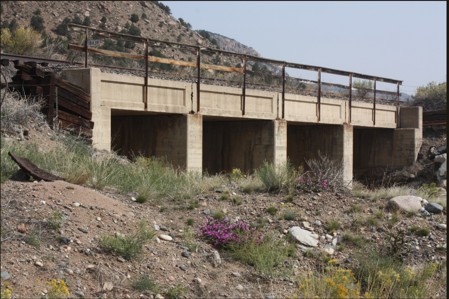
Northward view 200 feet southwest of the previous location where a bridge carries the D&RG Leadville Branch (1880n) over Texas Creek Gulch (not to be confused with Texas Creek [no "Gulch"], which is on the other [south] side of the Arkansas River).
