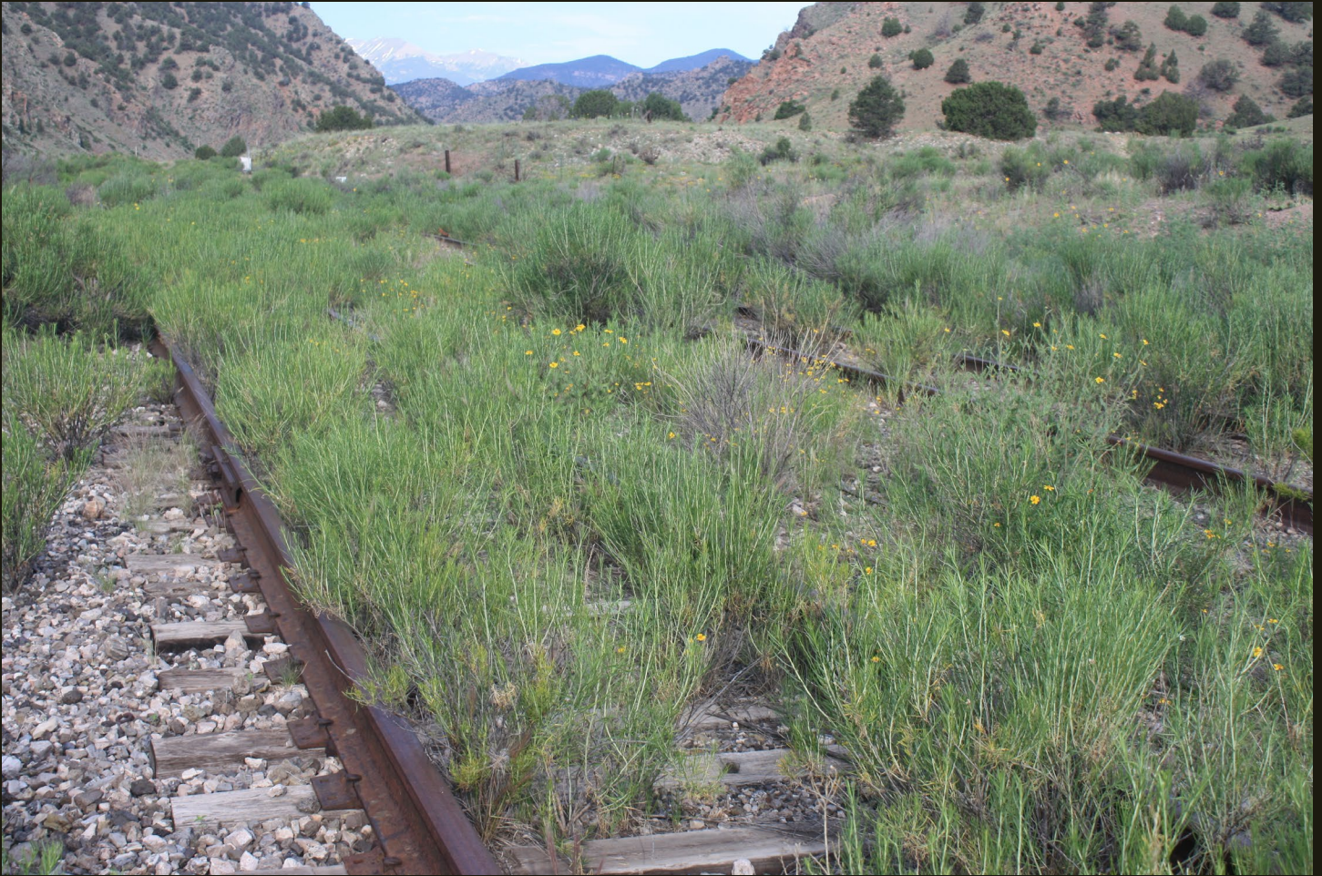
Westward view of the D&RG Leadville Branch (1880n) 100 feet southwest of the previous location. The 13,000-foot Sangre de Cristo Range, barely visible in the distance is not the Continental divide but does form the divide between the Mississippi and Rio Grande drainages.
