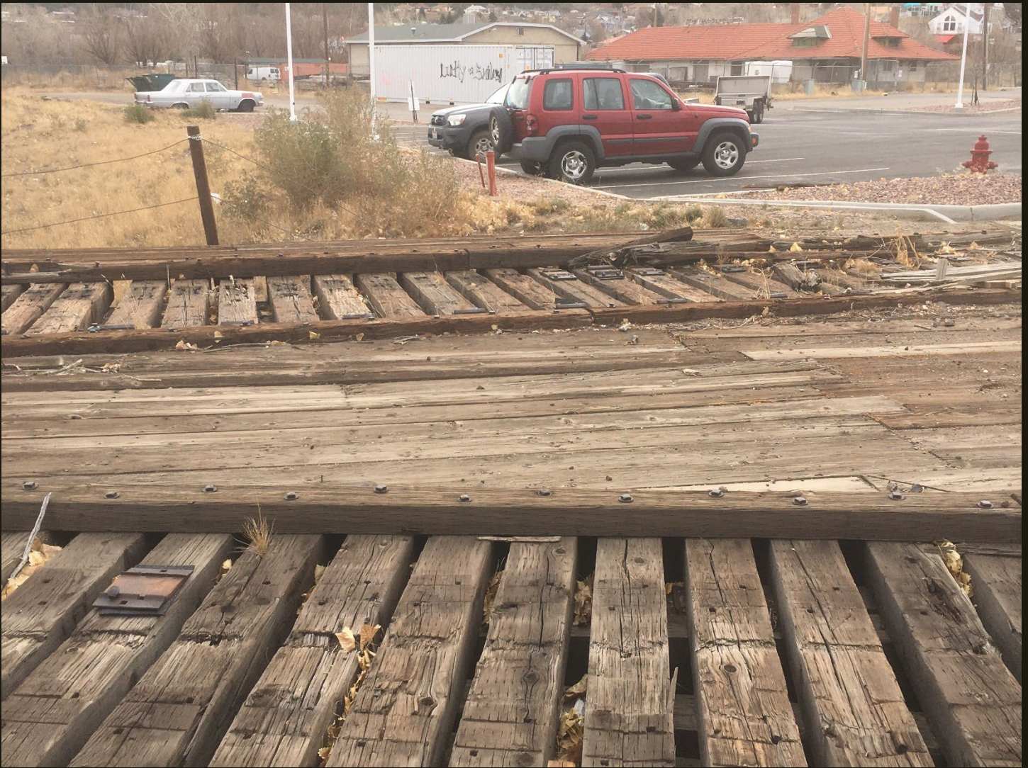
Southeastward view of the UPD&G (1895) second crossing (1895-ca 2000) of the Purgatoire River. The nearer track is the northwest branch of the wye, which continues southwest to the now-abandoned DT&FW Maxwell Branch (1888), and the farther track is the mainline to the DT&FW (1888) to Texas. Note the red roofed building in the upper right of the photo; it looks like a railroad station.
