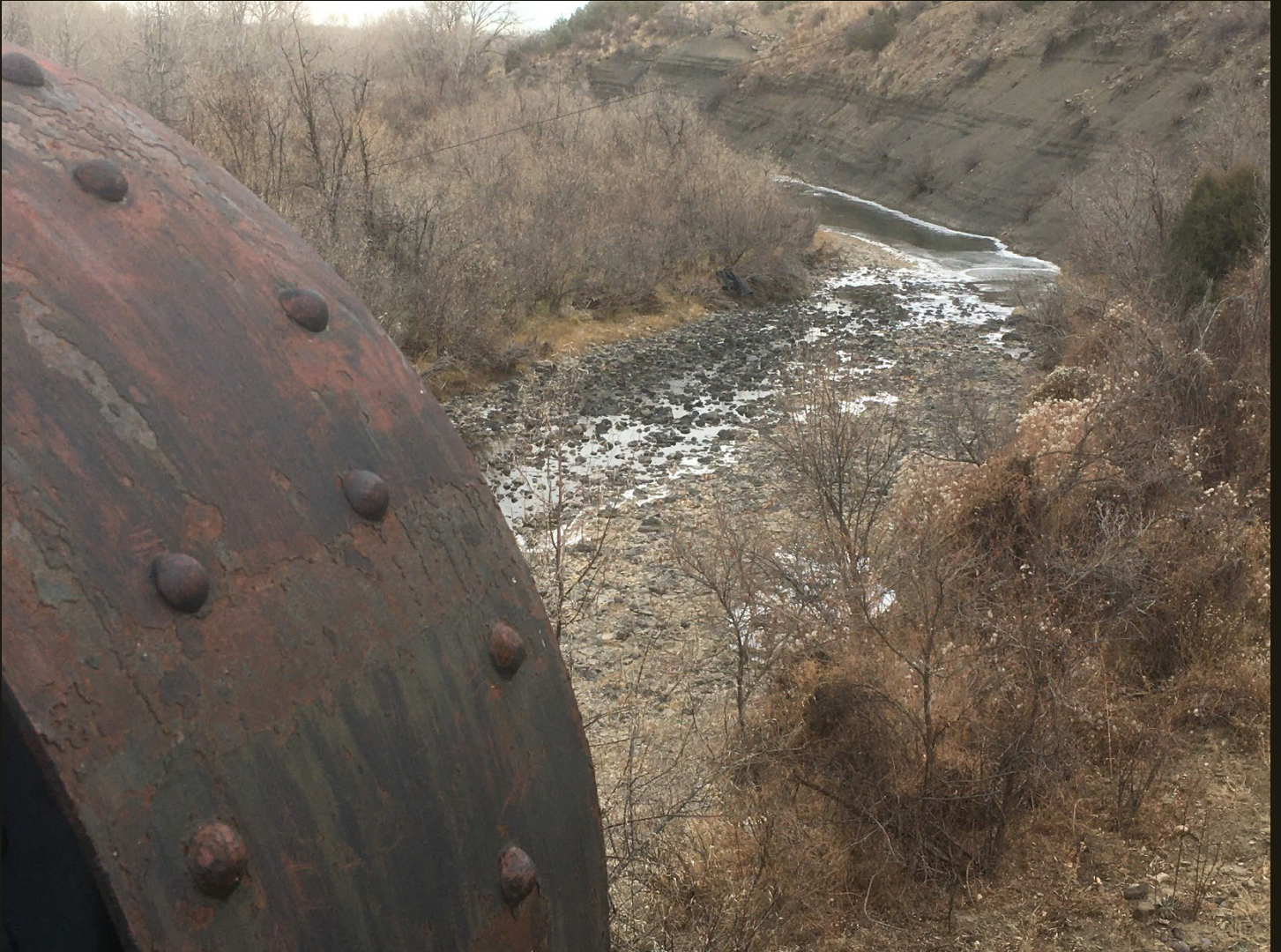
Eastward view of the south end of the bridge and the partially frozen Purgatoire River.
