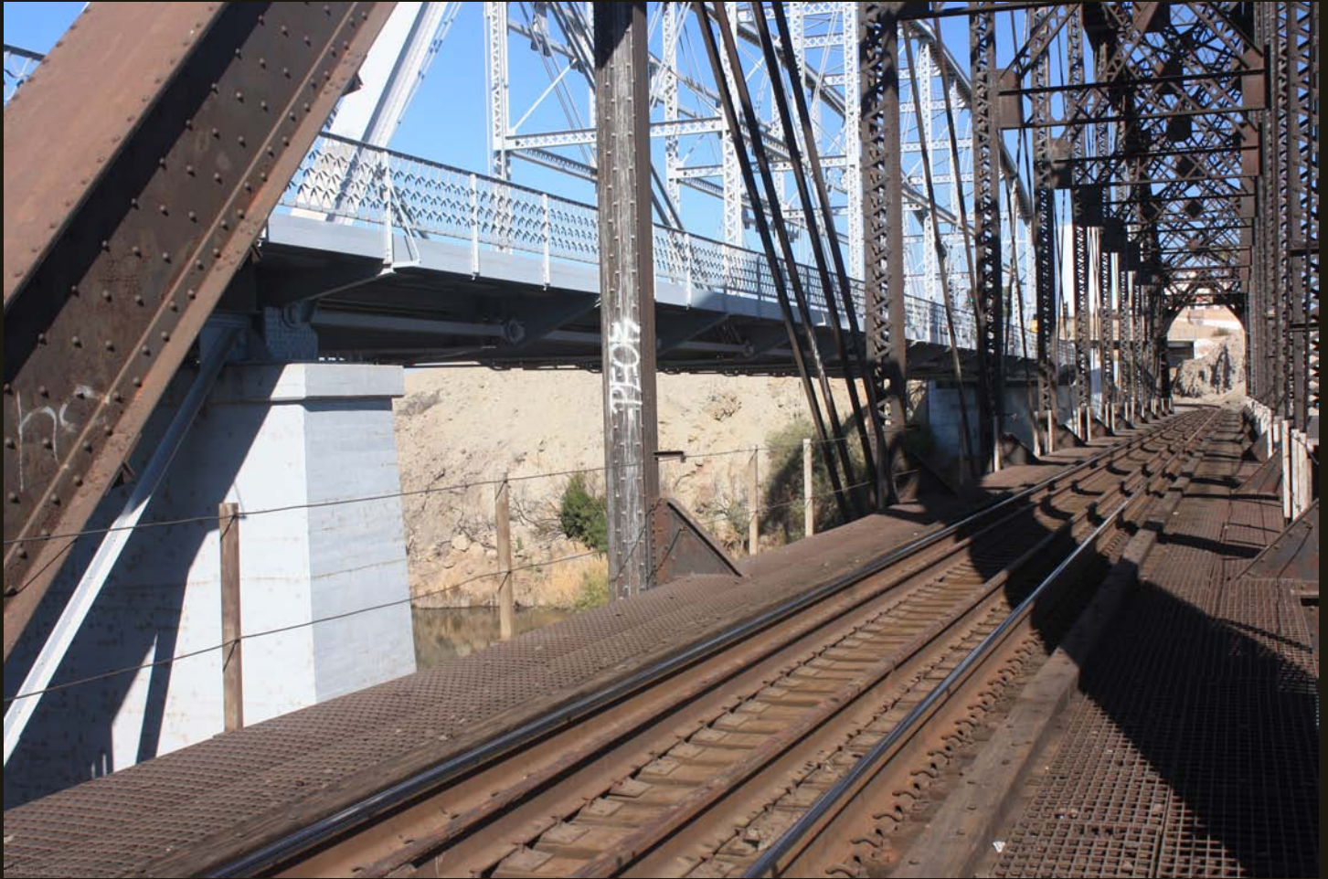
Closer view, in the westward direction, of the second SP bridge across the Colorado River at Yuma and the 1914 highway bridge next to it. Note the steep bank of the river, which keep it in a narrow channel at Yuma, and the cut in bedrock to maintain the rail grade on the far (California) side.
