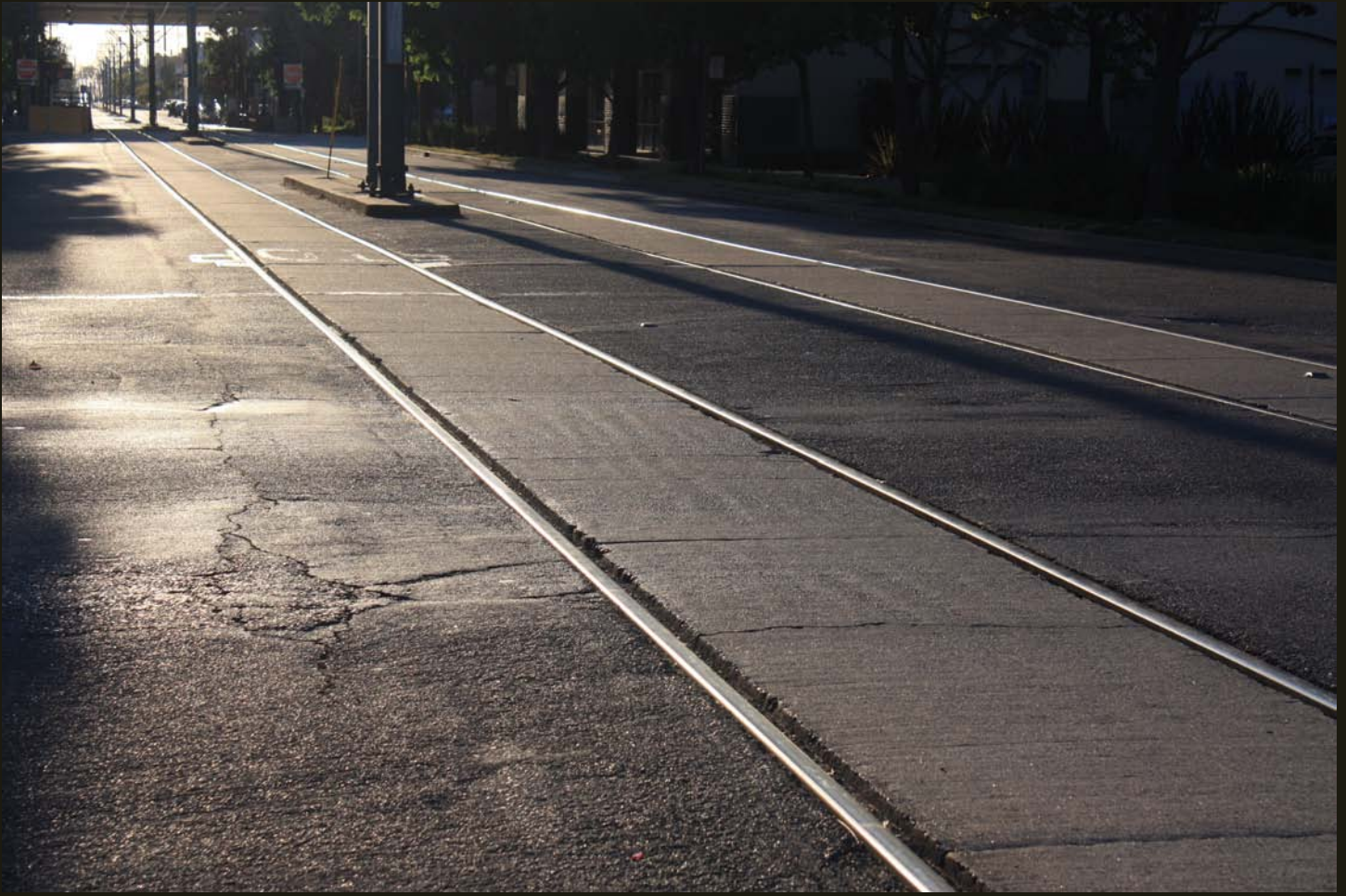
Westward view of R Street at Alhambra Boulevard (which could have been called 31st Street), showing Gold Line tracks on the SV alignment. This is the easternmost location where the SV alignment is in R Street.
