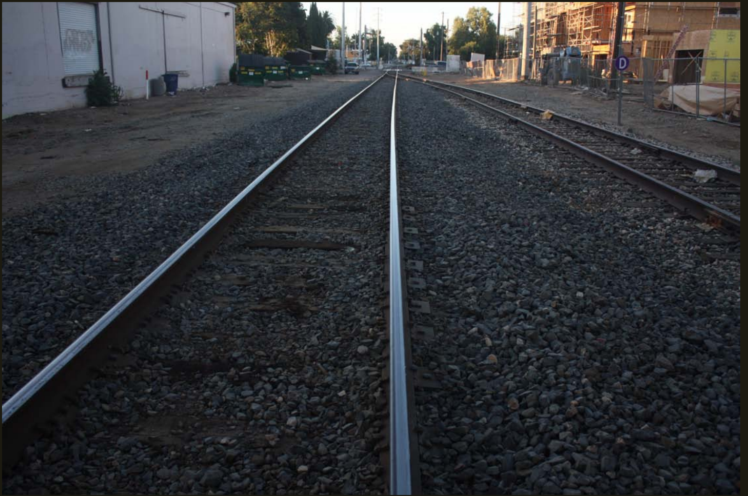
Northward view of the WP (1909) converging to a single track, same location as previous.
