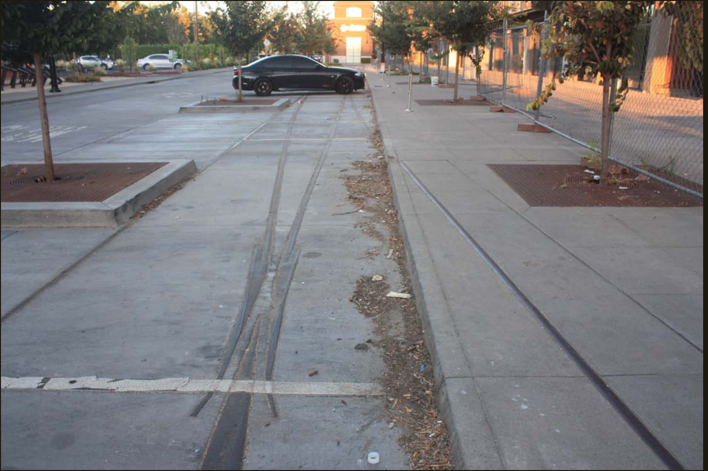
Westward view on R Street, just east of 17th Street, showing detail of an old switch. Note the red brick building in the distance; it is on 18th Street and the tracks and R Street end there, removed for retail development.
