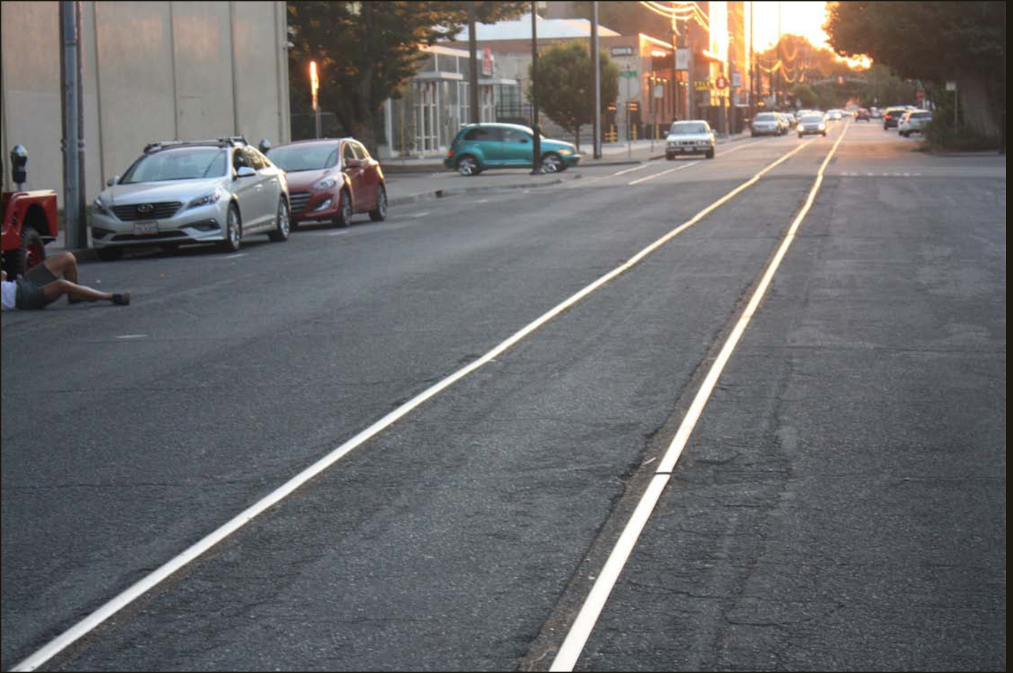
Westward view of the SV/S&P/SP/UP trackage on R Street, just west of 14th Street. These tracks are as the SP left them -- note there is a place for the flange of a wheel.
