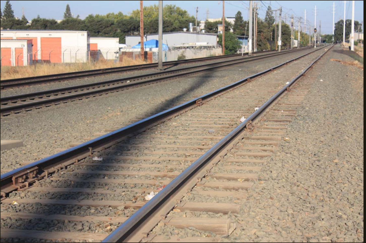
Eastward view of the SV (1856) alignment, same location as previous. The UP tracks are on the right and continue to the Aerojet facility just west of Folsom, and the Gold Line tracks are on the left and continue to Folsom at the original SV (1856) end-of-track.
