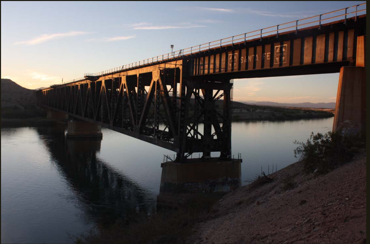
Westward view of the 1945 AT&SF bridge over the Colorado river at Topock.
