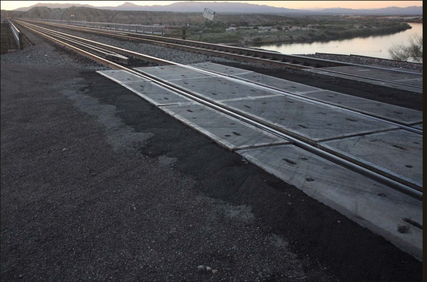
Another view of the 1945 AT&SF bridge over the Colorado River at Topock, looking westward from Arizona.
