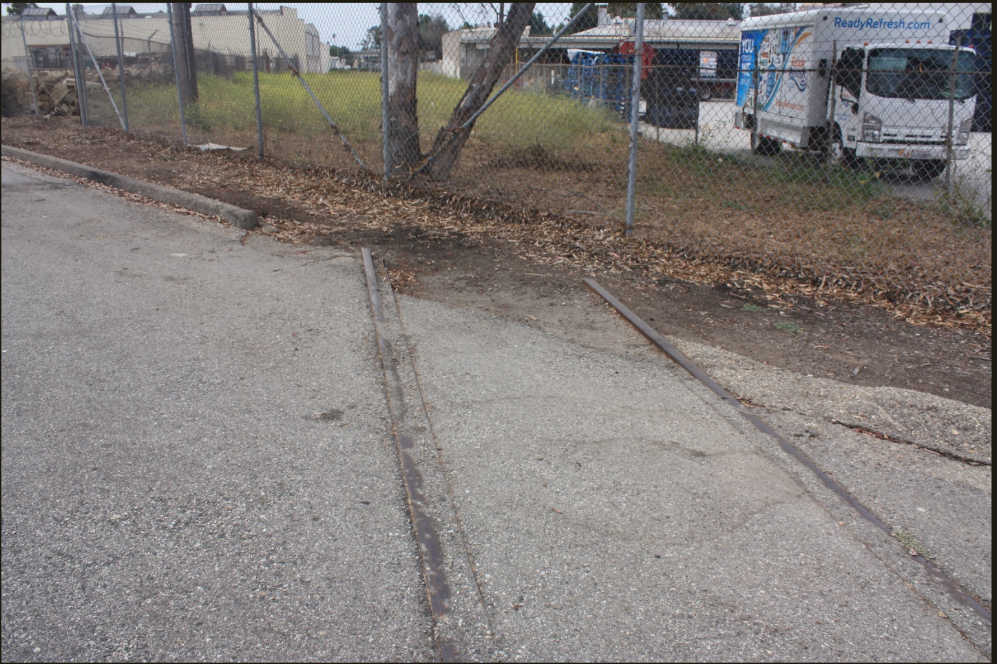
Southward view of the V&OV (1898) at the same location as previous. The vacant area behind the tree extends 500 feet south and all traces of the remaining 1,500 feet of the V&OV (1898) south this vacant area, including the junction with the SP mainline, have been obliterated.
