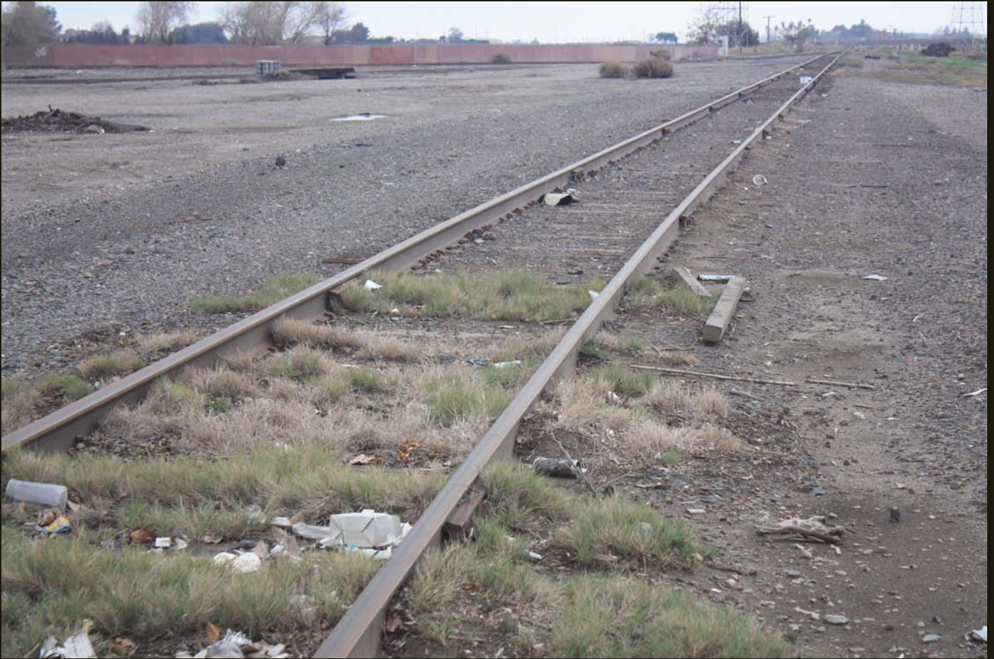
A few steps farther southeast within the wye for the SP West Side Line (1891) looking southeastward. The straight track in the foreground is the old alignment of the SP West Side Line (1891) and the curved track that merges with it in the distance is the east branch of the larger wye. The west branch of the wye merges with the straight track just out of sight in the distance.
