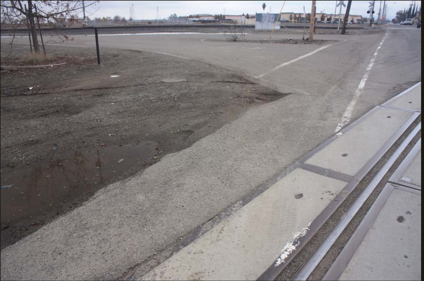
The puddle in the left foreground is the same one as in the previous photo. Note the curved right-turn-only road, which is unusual for this minor side street and could mark the prior alignment of the east branch of a wye for the spur.
