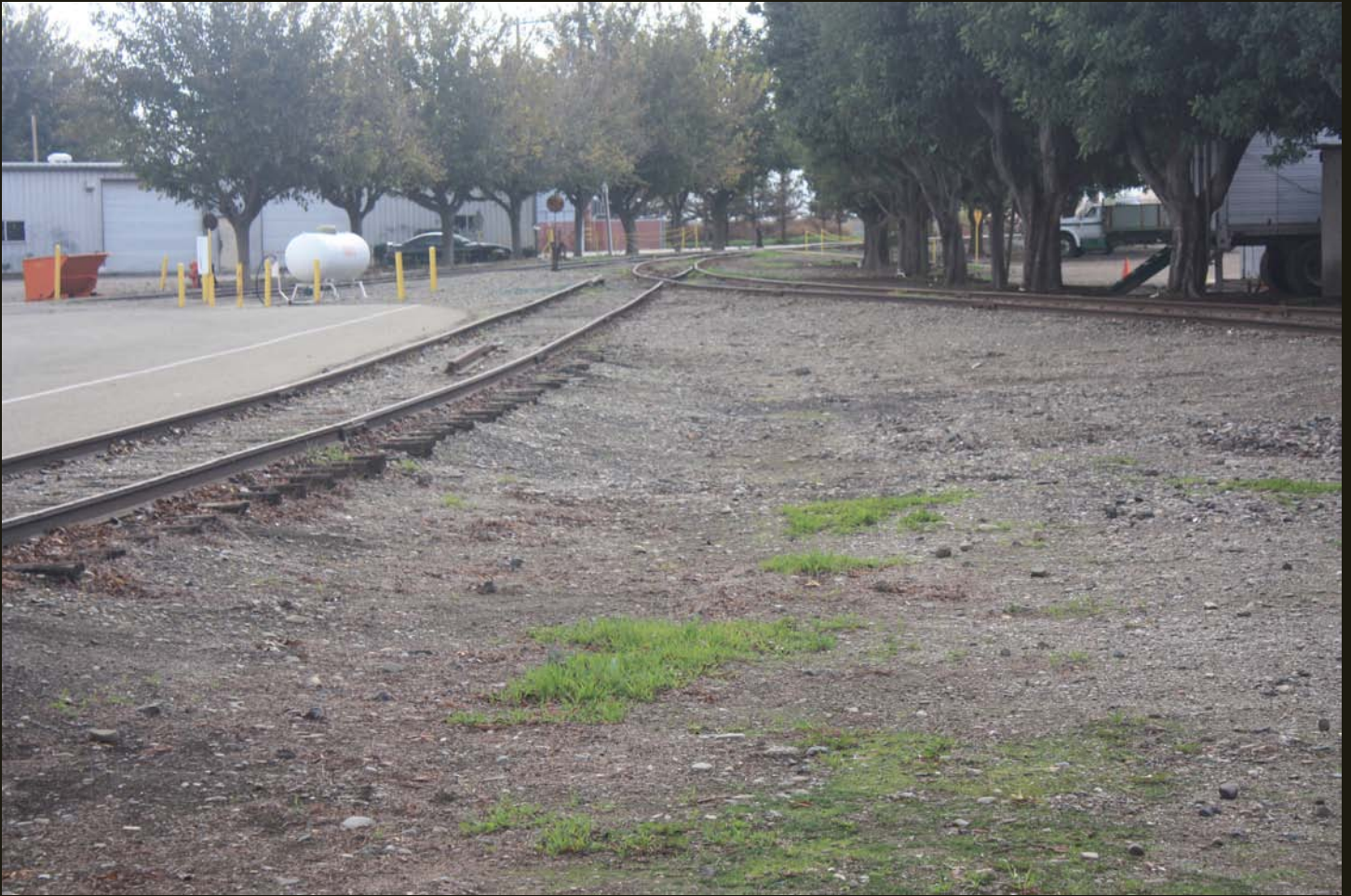
In this southward view, the near switch with missing track is the tip of the wye connecting the WP (1909) with the Tesla Branch. The farther switch is a spur to some warehouses, and beyond that the track curves southwestward (to the right) onto the A&SJ (1896) alignment (previous photo).
