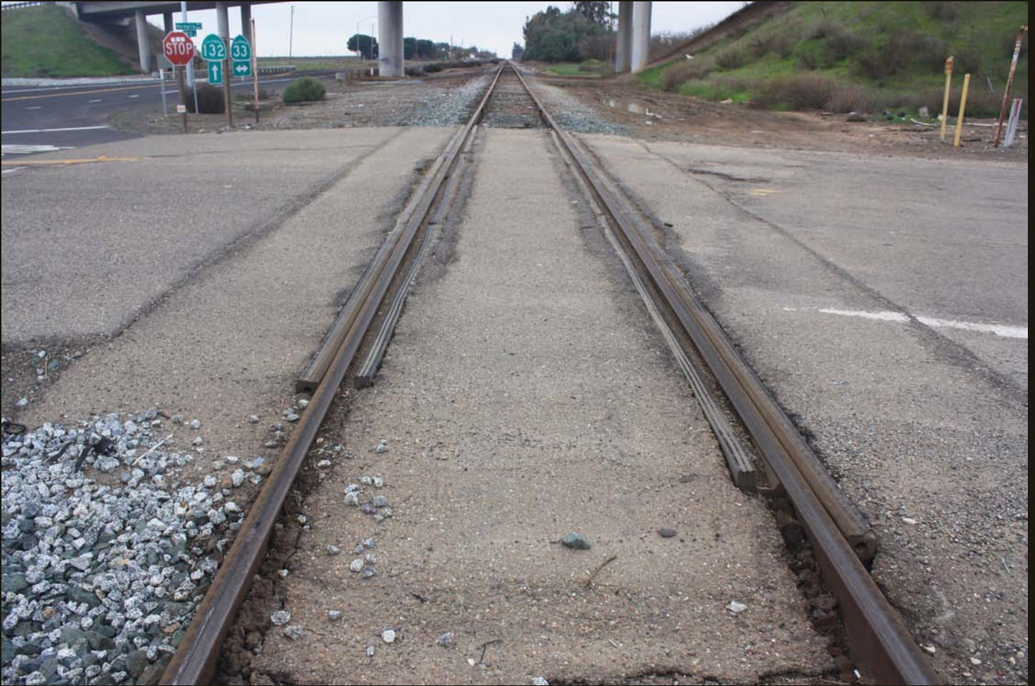
Southeastward view of the SP West Side Line (1891) (now California Northern), same location as previous (10 miles southeast of Tracy), where the line passes under California Highway 132. The line continues another 50 miles to Los Banos, beyond which the West Side Line tracks are gone.
