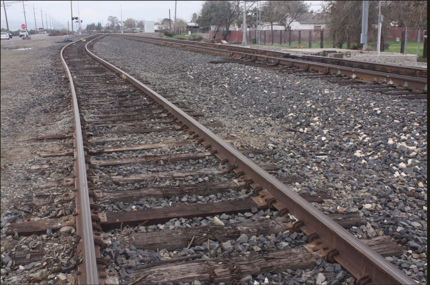
Westward view of the west end of the Carbona wye, same location as previous. All tracks converge to one track in the distance.
