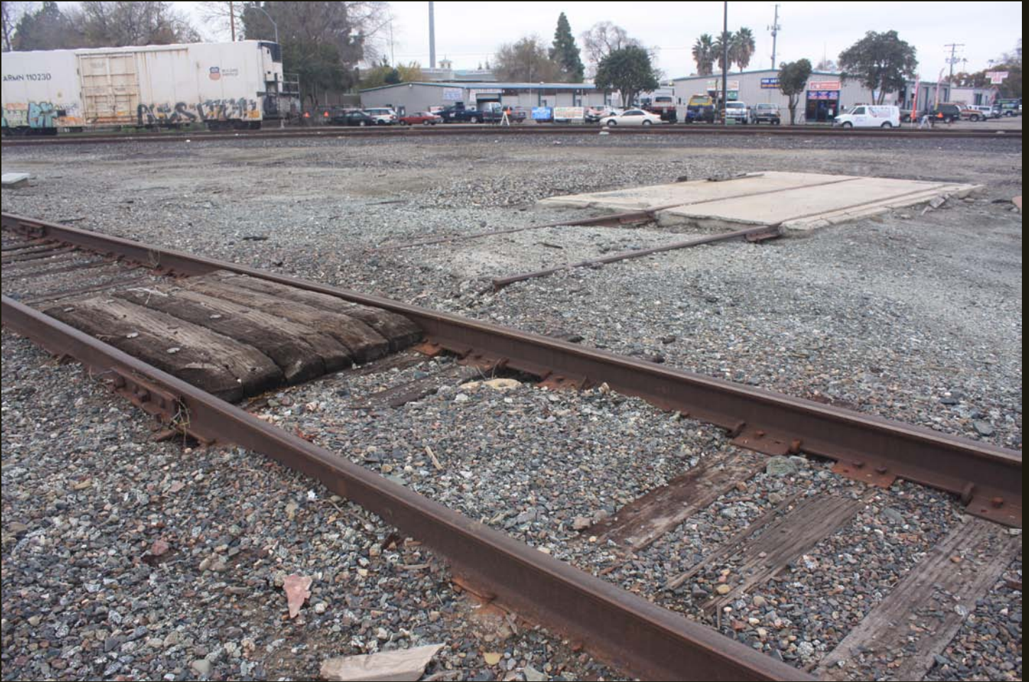
The west branch of the wye for the SP West Side Line (1891), with some sort of an old track-side foundation. The UP box car is on the WP (1869) siding. Note the rusty track; there is really no place worth going westward from here by rail.
