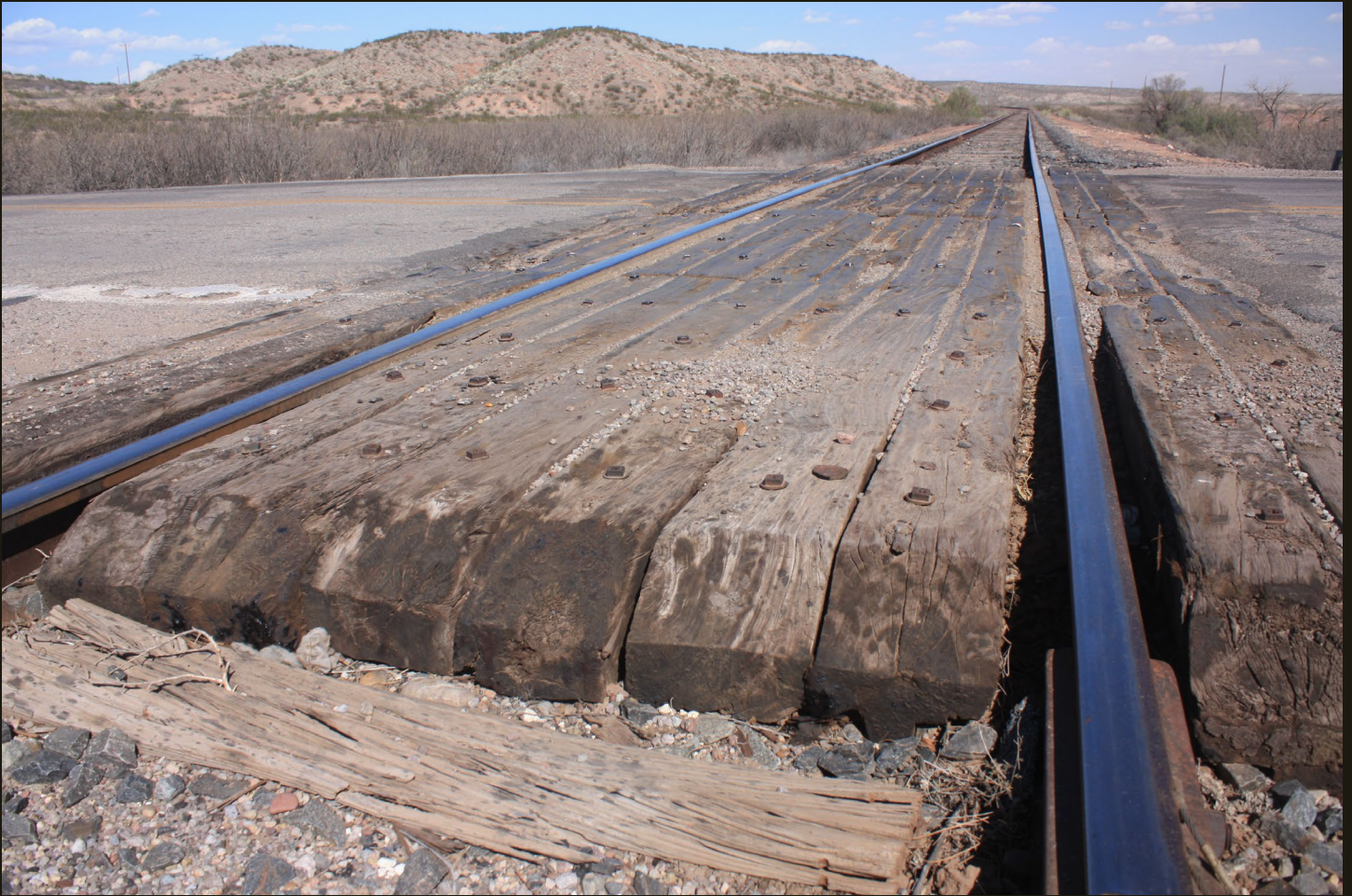
Road crossing of the AT&SF's RGM&P (1881) line to Deming where it leaves the Rio Grande Valley southwest of Rincon. In 2001, the Southwestern Railroad acquired the RGM&P (1881) from Rincon to Deming from BNSF.
