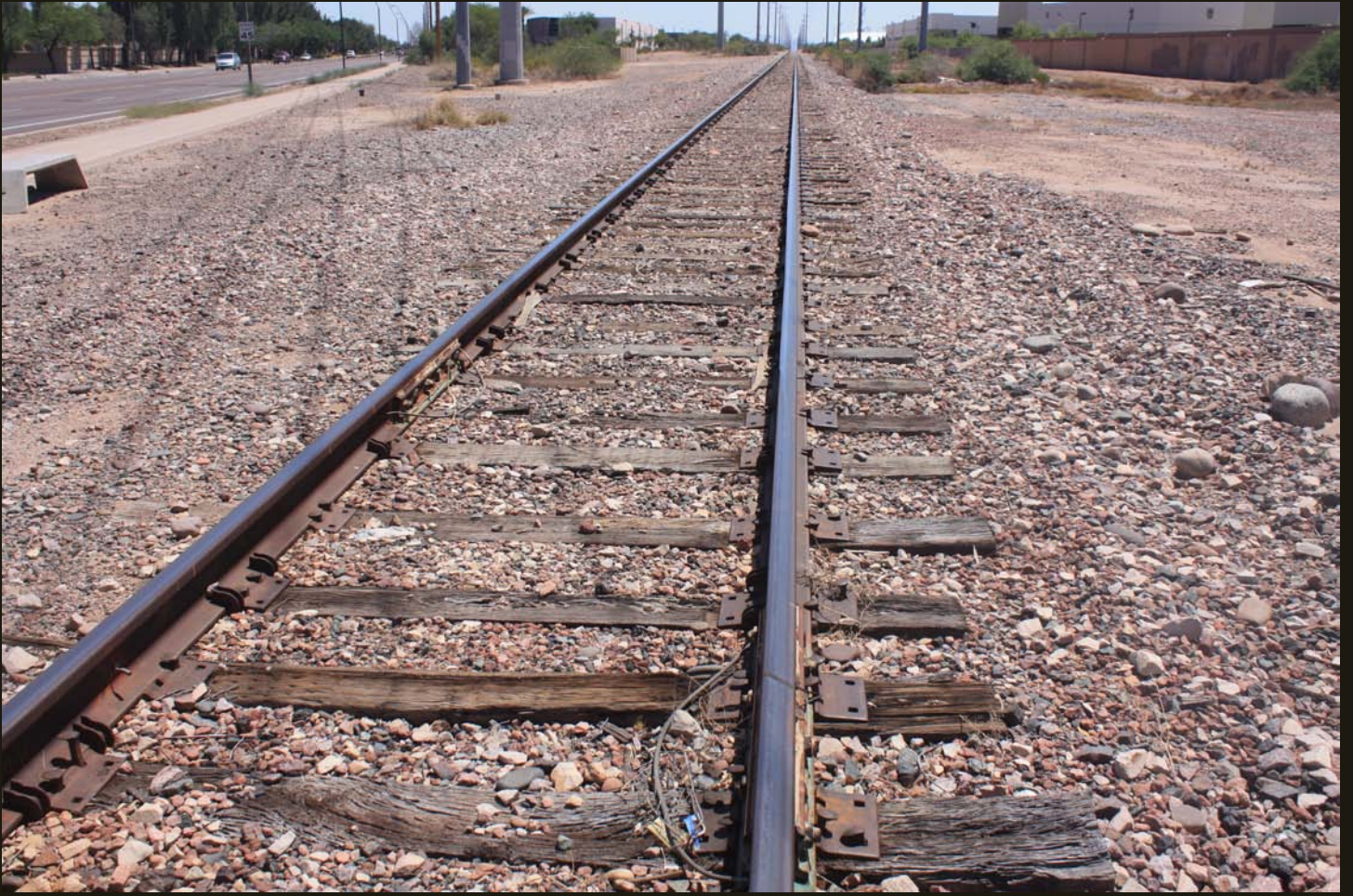
Southward view 5 miles north of the current end-of-track (previous location) and 5 miles south of Tempe on the M&P (1887) grade.
