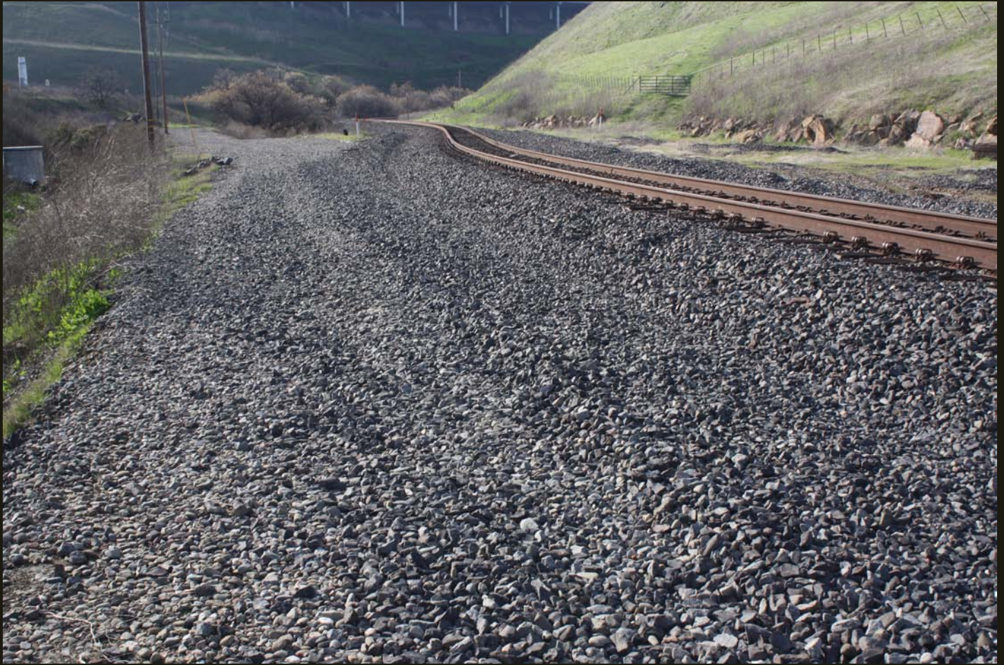
Southwestward view a few steps up the grade from the previous photo. The abandoned WP (1869) grade and the WP (1909) tracks appear to merge. The bend in the WP (1909) tracks suggest that it was re-aligned to utilize the abandoned WP (1869) grade.
