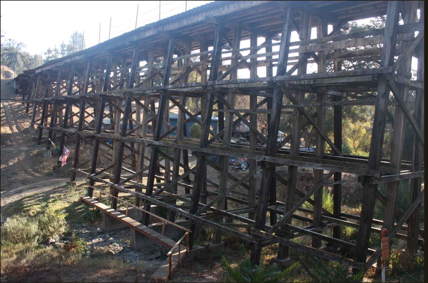
Eastward view of the trestle that carries Cement Plant Road over Willow Creek. The 1935 concrete bridge and Highway 49 are just out of view on the right. It sure looks like a railroad trestle!
