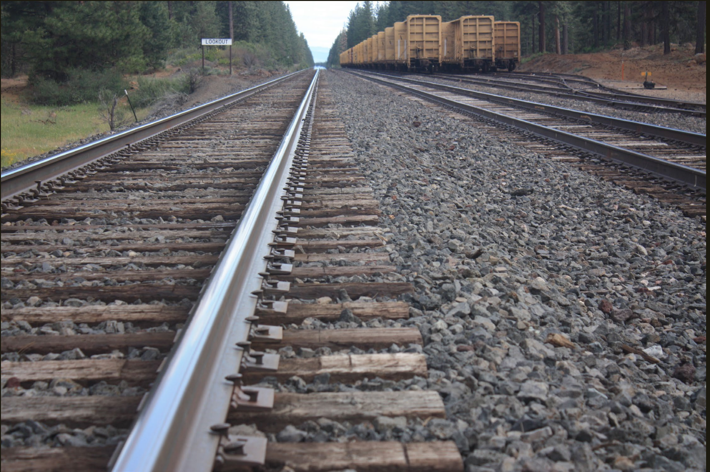
Now we are back at the GN Inside Gateway (1931) mainline looking south at the same stored cars. From left (east) to right the tracks are: the Inside Gateway (now BNSF) mainline; the primary siding (for passing trains); and the loop line track (Hamburg Branch, with stored cars on it) and two additional sidings for car storage.
