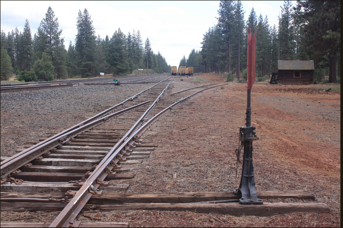
Southward view a few steps north of the previous location showing the same disconnection. Note the same shed and stored cars as before.
