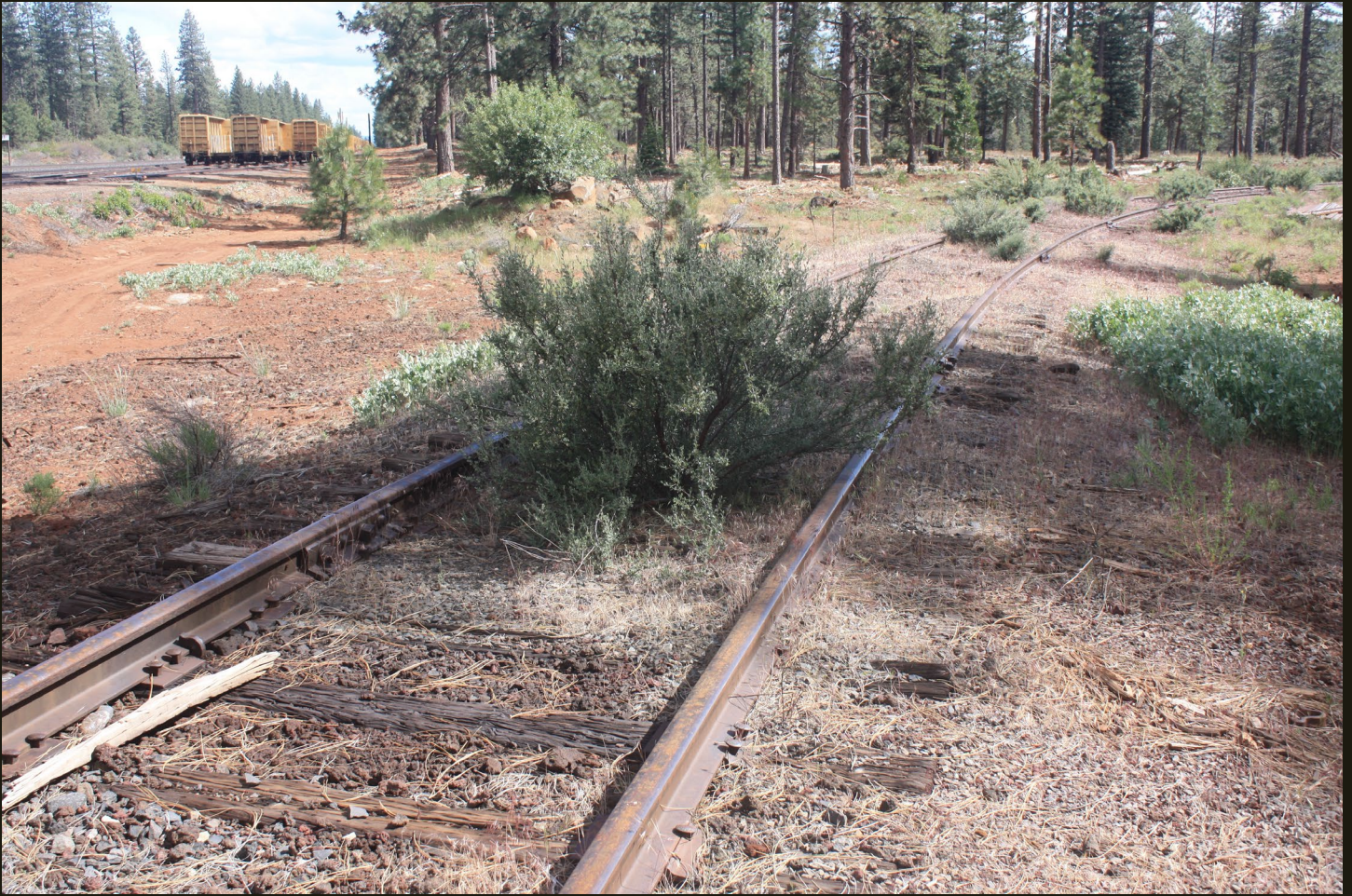
Southward view of the loop track 200 feet south of the shed. Note the same stored cars on sidings of the GN Inside Gateway (now BNSF) mainline.
