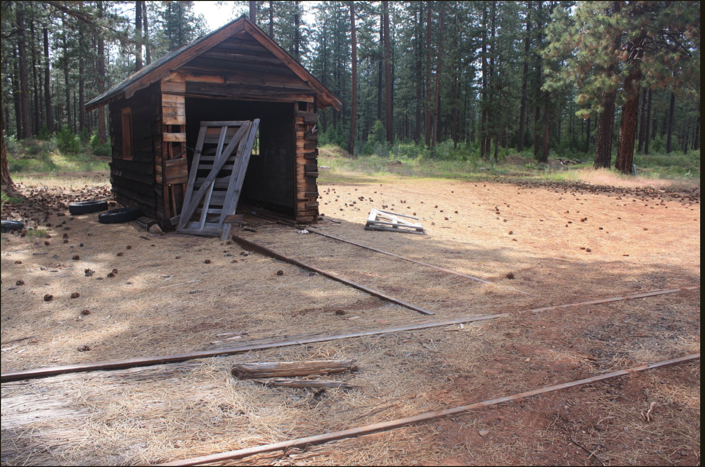
Westward view of the shed at Lookout Junction. The track in the foreground is the GN Hamburg Branch loop track. I assume the shed is some sort of maintenance shed and I've seen similar sheds with rails between the track and the shed, but I don't know what the rails are for. Maybe some sort of cart was run on the rails or maybe the rails are just to establish a pathway.
